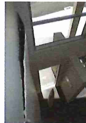
Significant sheet fracture
