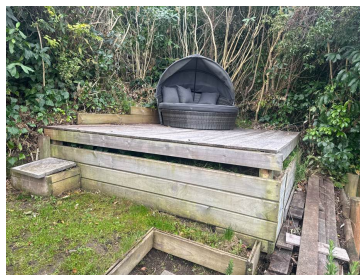
This platform needs a handrail, straightening underneath, steps
