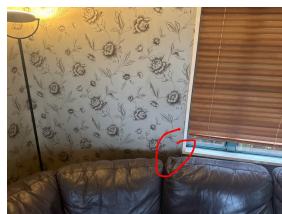
Elevated moisture readings in this corner
