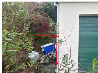
All downpipes directed into stormwater as intended
