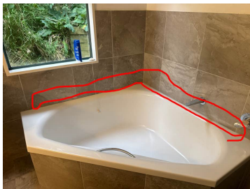
Hi moisture detected in these areas
