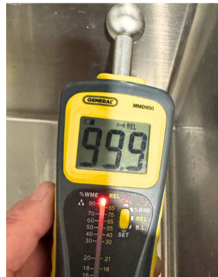
High moisture reading: Red: Damp = 20+ Wet = 50+
