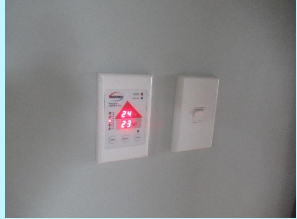
Heat recovery and ventilation system control panel
