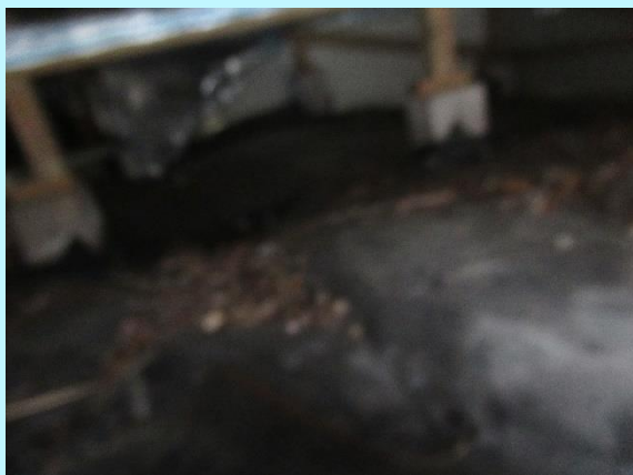
A ground vapour barrier is fitted to inhibit rising damp and moisture below the dwelling
