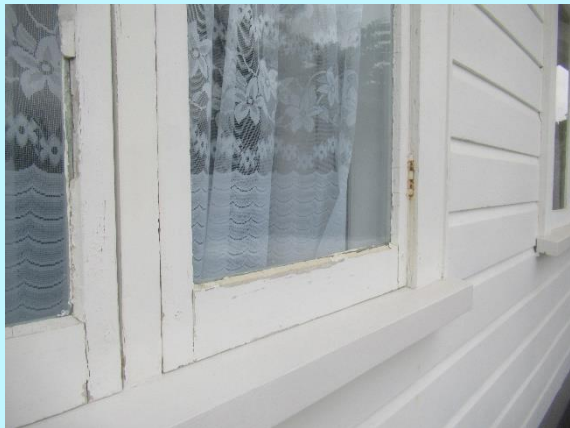
Deterioration and missing glazing putty in the windows are now due for renovation and repairs
