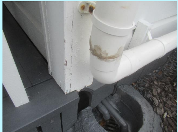
Deterioration and some decay in the external trims that will require ongoing maintenance and repair
