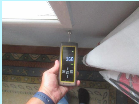
Dry moisture readings located around bedroom 4 window
