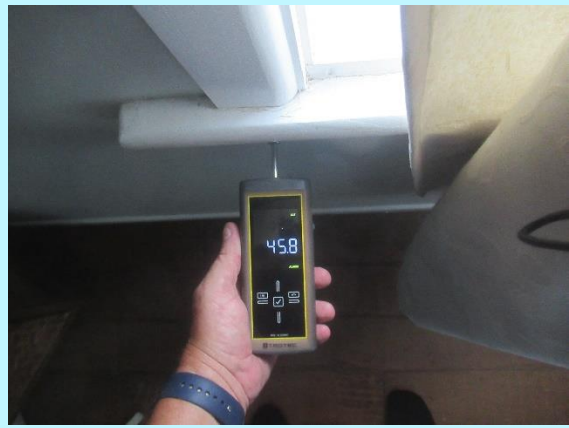
Dry moisture readings located around bedroom 1 windows
