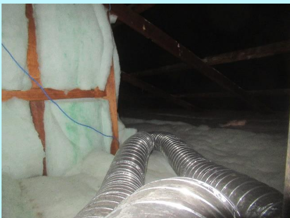
The walls and ceilings are correctly insulated around the bedroom with a sarked skillion roof
