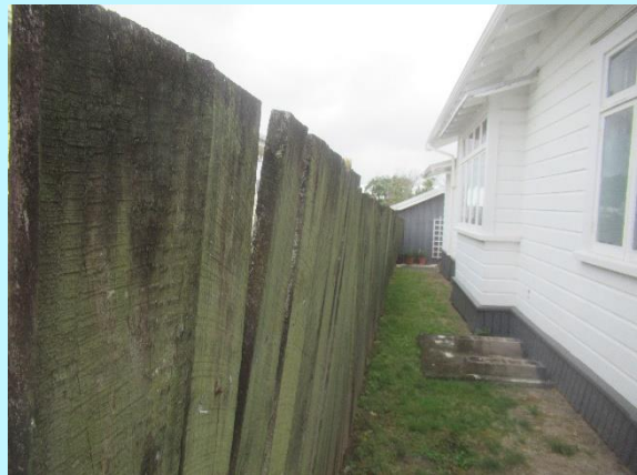
The timber fencing at the boundary has failed and is leaning into the property
