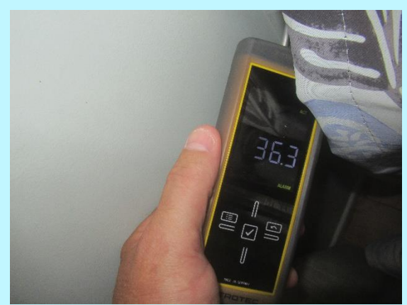
Dry moisture readings located around the lounge windows and walls below the flue
