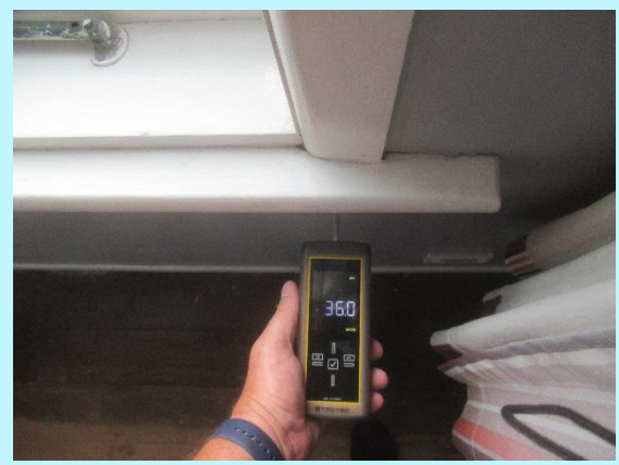
Dry moisture readings located around bedroom 2 window
