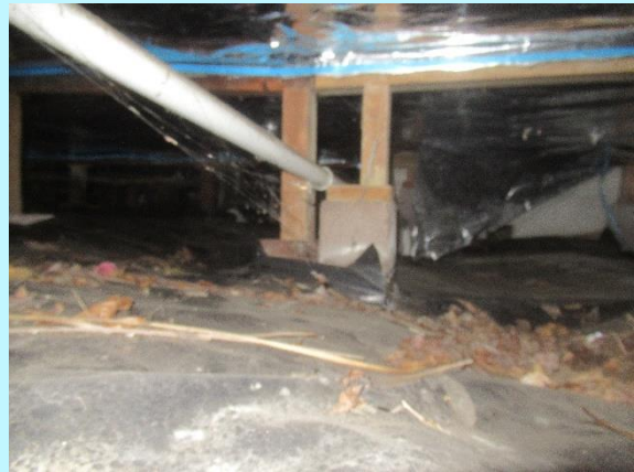
The visible subfloor framing is original and is dry and well ventilated with no significant issues seen
