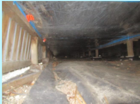
The concrete piles indicate a full re-pile, we did not feel any obvious deviation in the floors underfoot
