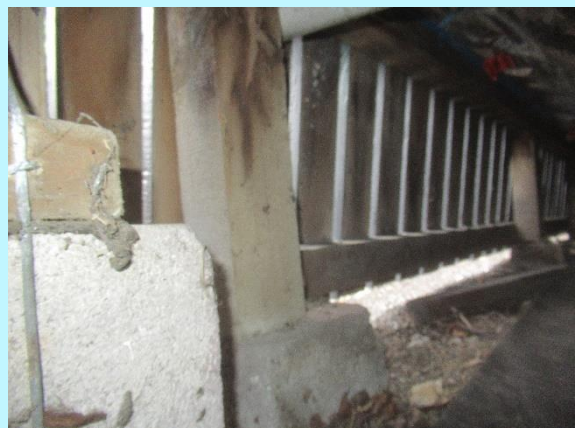
The dwelling appears to have been replied, we cannot verify the size or suitability of the footings
