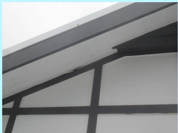
The timber soffit lining is deteriorated the soffit are reasonable however maintenance is needed
