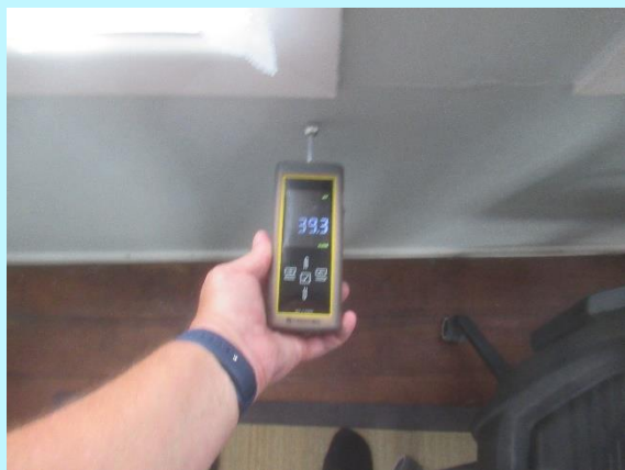
Dry moisture readings located around bedroom 3 window
