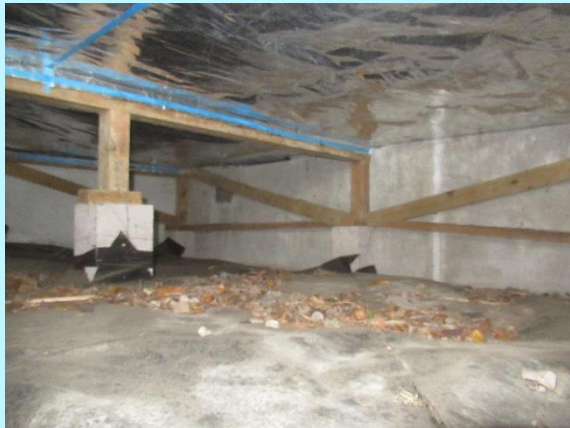
concrete piles with timber jack studs provide the foundations, the dwelling has been re-piled
