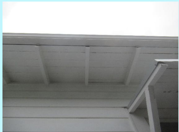
Exposed outriggers and timber sarking soffits are reasonable with no significant defects noted
