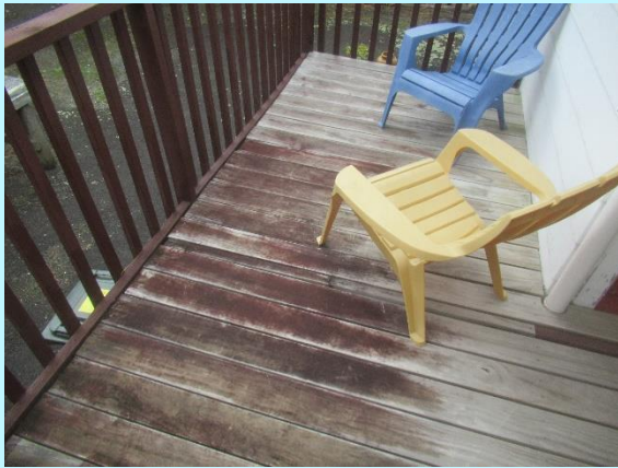
The front and rear decks are due some work around the foundations and jack framing
