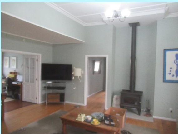
Lounge with free standing wood fire installed as the fixed heating and cooling
