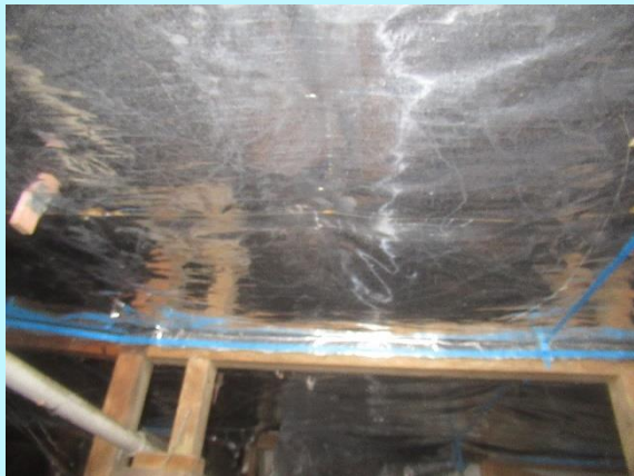
The subfloor is fitted with foil insulation which prohibits a view of the underside of the flooring
