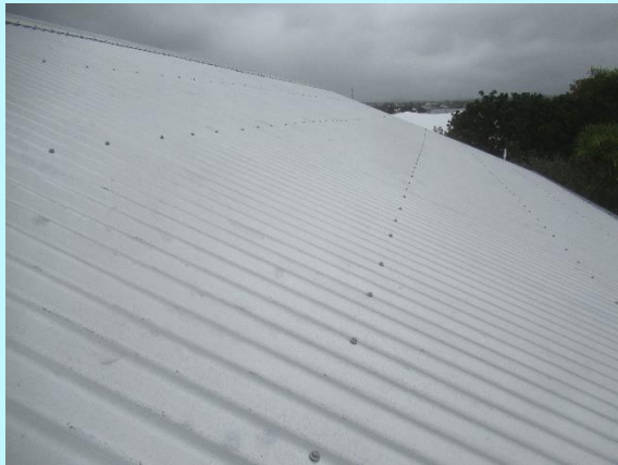
The corrugated roof is a reasonably new and is suitable for the design, location and wind zone
