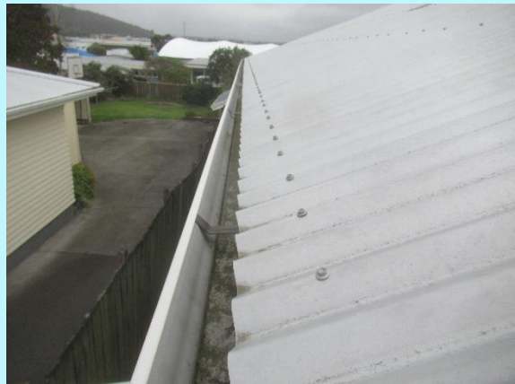
The external Upvc gutters are clean and clear with suitable fall to the outlets
