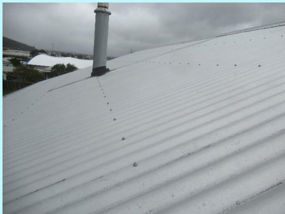
Back soakers trays, apron, ridge and hip flashing are securely fixed and suitable for the roof
