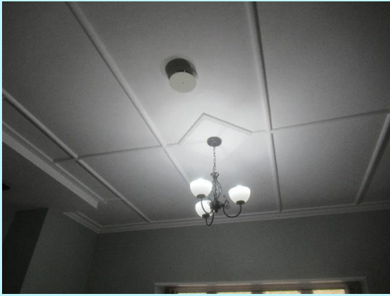
Timber batted ceiling linings with diffuser providing filtered dry air into the dwelling
