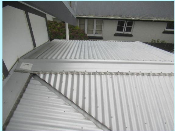
The roof should be cleaned and chemwashed to inhibit lichen growth and preserve condition
