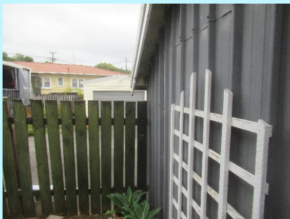
This ancillary building is on the boundary and is discharging water runoff to the adjacent dwelling
