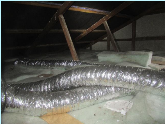
A ventilation and heat recovery unit is installed to provide positive dry air pressure into the dwelling
