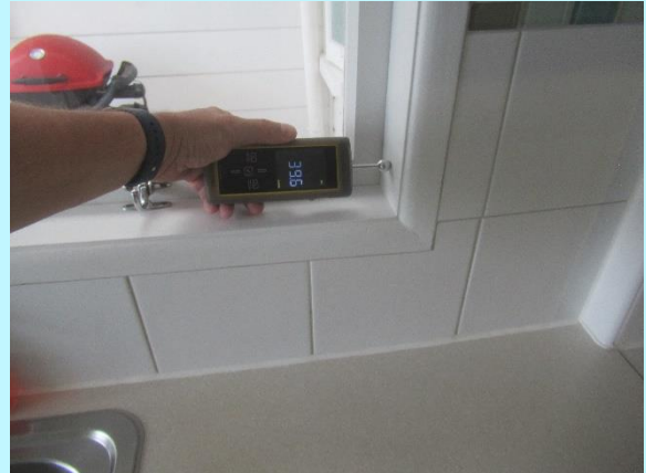
Dry moisture readings located around the kitchen windows and cabinetry below the sink
