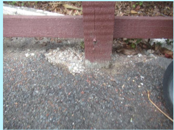
Decay and out of plumb piles noted below the rear elevation decks, repairs are due soon
