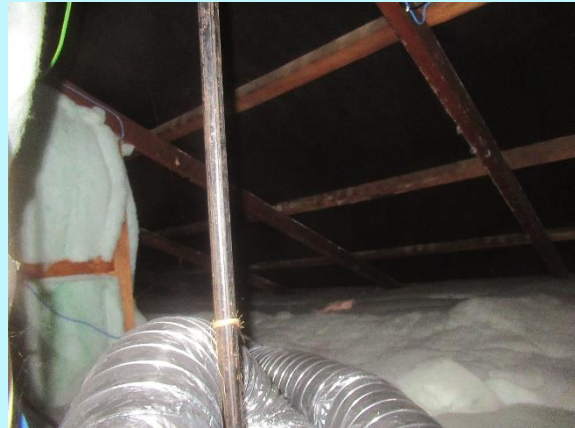
Building paper is installed to control condensation from the underside of the new profile metal
