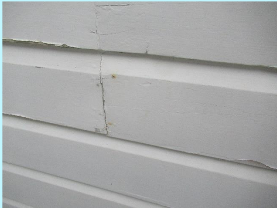
The cladding is original with some splitting and deterioration consistent with age and wear
