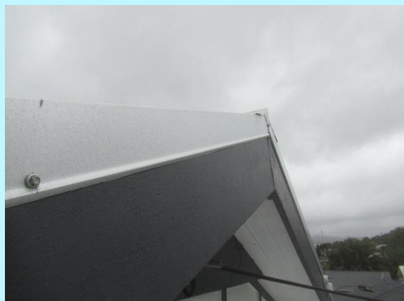
The barge and ridge flashings are secure, and the soft edges are moulded down to the roof surface
