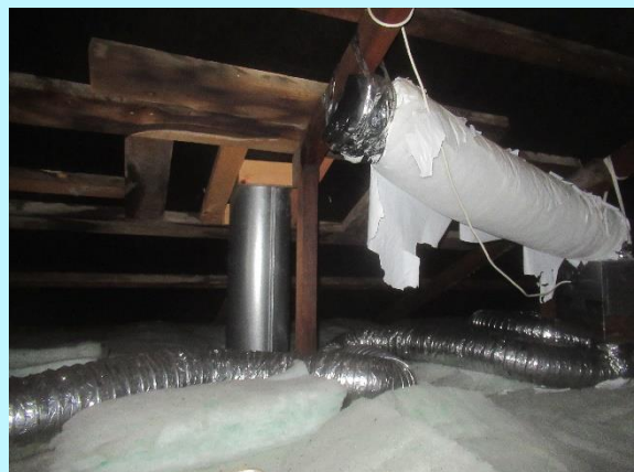
Our inspection is visible and from the access hatch we do not enter the roof cavity
