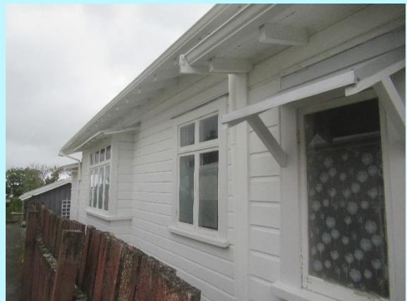
Western side elevation with damaged fencing and ancillary dwelling against the boundary
