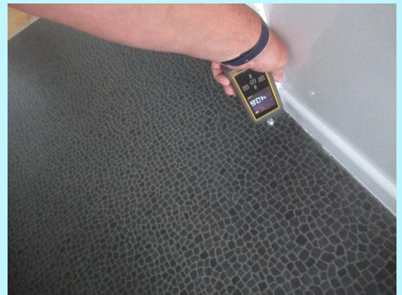
Dry moisture readings located at the bath to wall junction indicating the liner is correctly sealed
