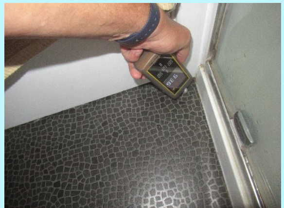
Elevated moisture at the shower to wall junction can indicate the liner is not correctly sealed here
