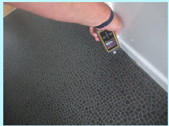
Dry moisture readings in the flooring indicate no leaking from the cylinder or valves in this area
