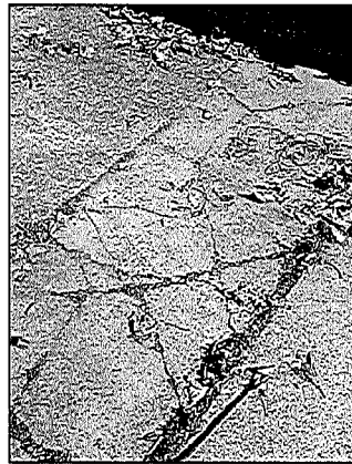
Photo 3: Cracking in driveway
