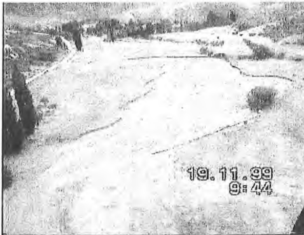
Middle reaches of proposed subdivision shows bank erosion
