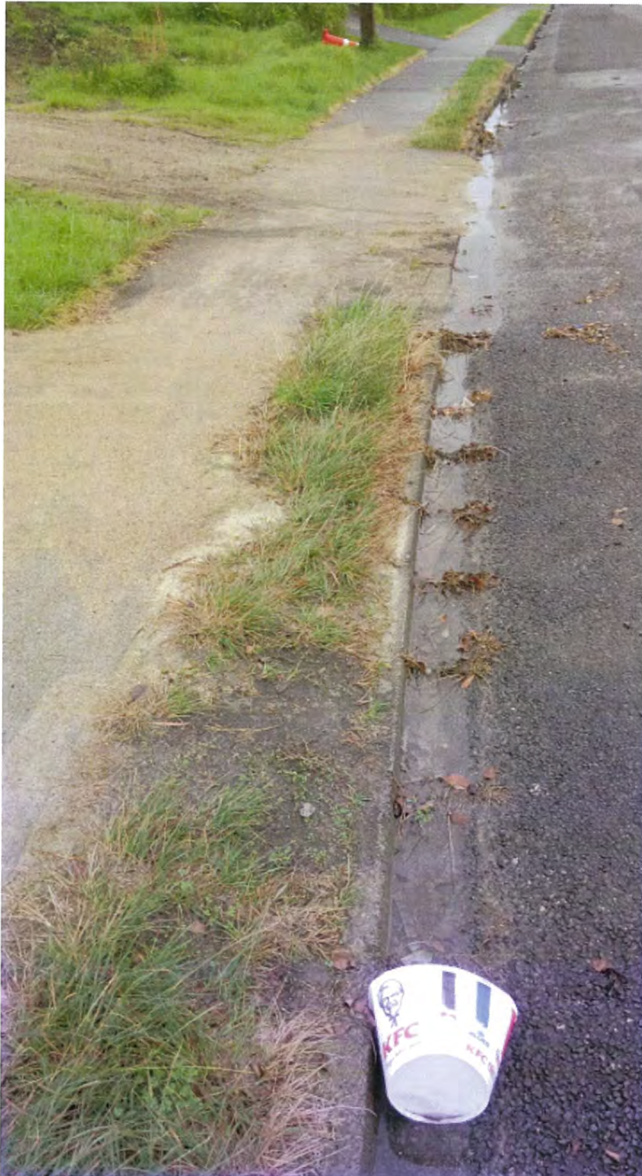
Figure 4: Photo looking west along footpath from street frontage of 5A Toi Street showing sediment from the site spilling onto the road reserve and into the stormwater system. Taken 17 May 2017.
