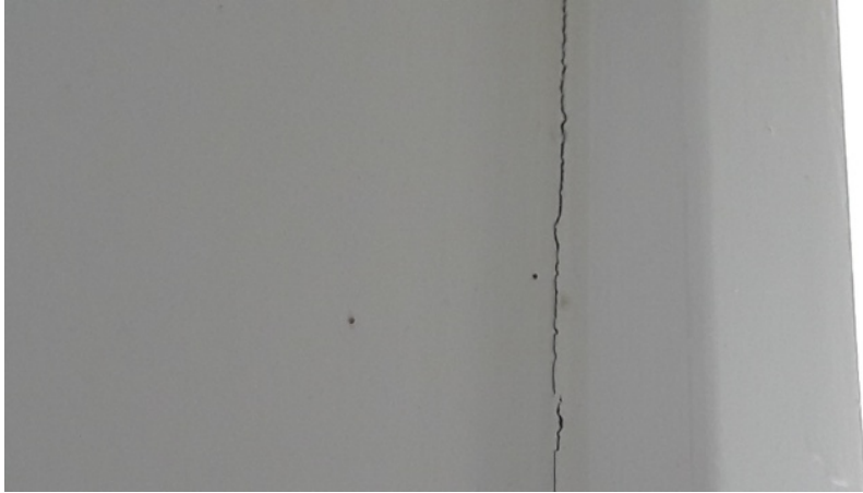
Figure 4 : Kitchen/Dining/Lounge jamb movement
