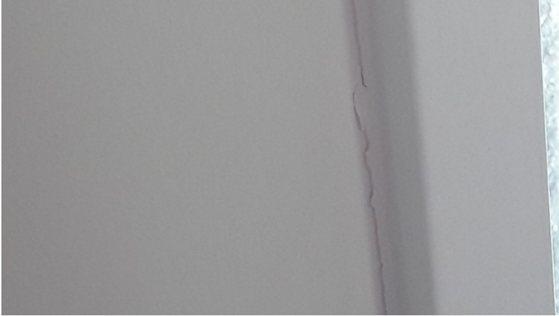
Figure 10 : Garage wall crack
