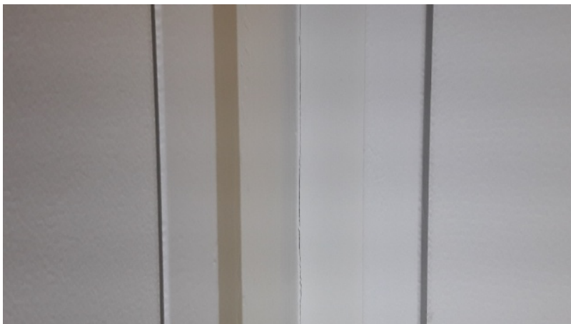
Figure 6 : Hallway wall cracking
