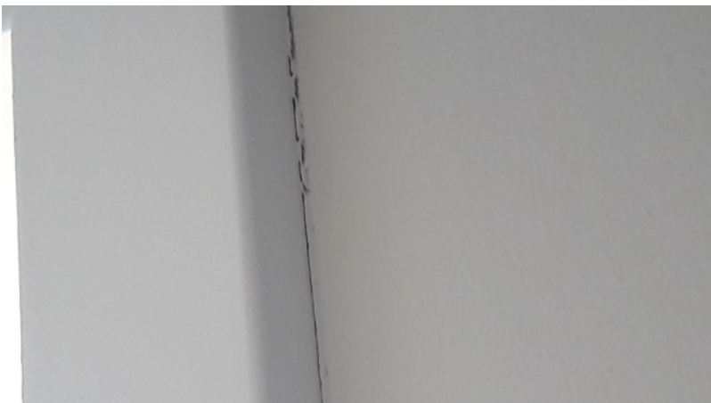
Figure 12 : Bedroom 2 jamb movement
