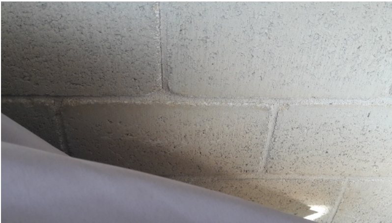
Figure 17 : Brick step cracking
