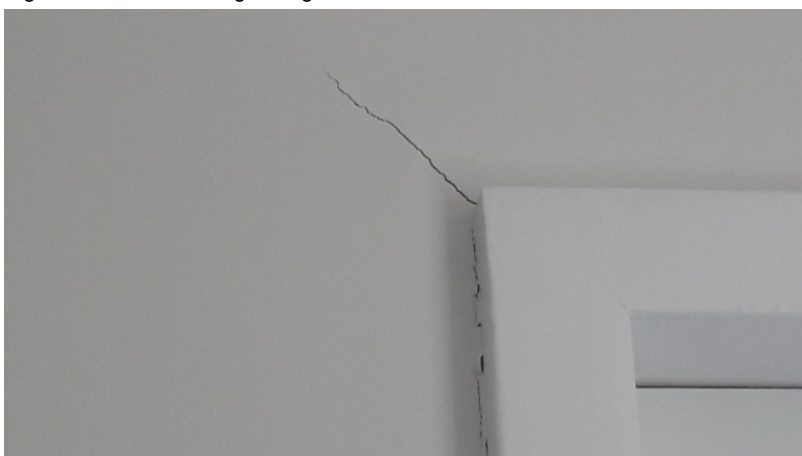
Figure 3 : Kitchen/Dining/Lounge wall crack
