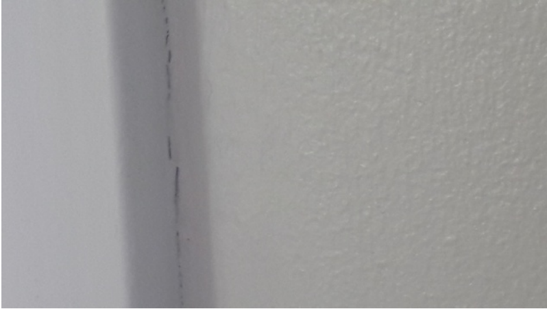
Figure 16 : Ensuite jamb movement
