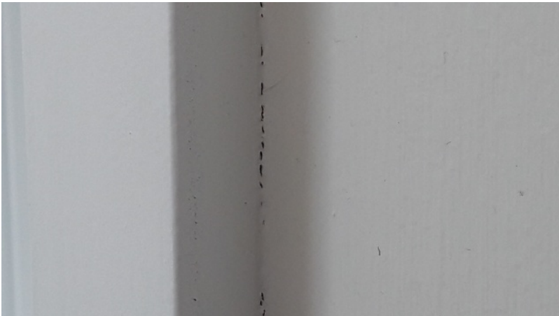
Figure 14 : Master Bedroom jamb movement
