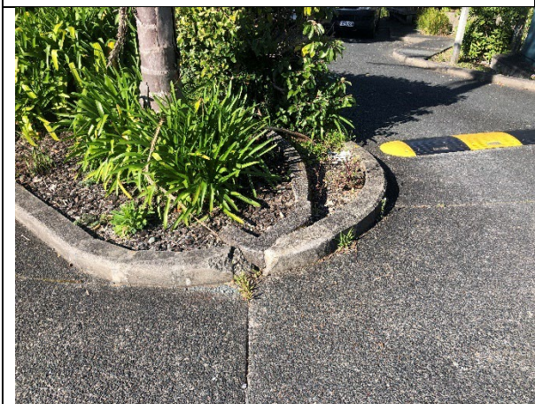
EXAMPLE OF DAMAGED KERBING, PU-23
