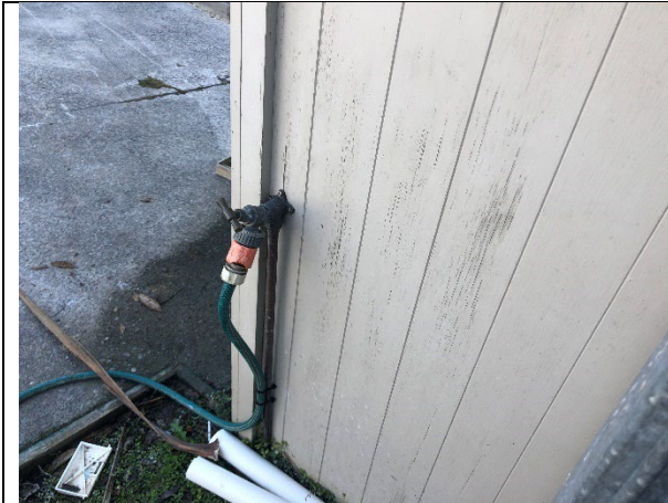
POOSIDE WATER TAP REQUIRES A VACUUM-BREAK TO BE INSTALLED (VERY INEXPENSIVE BUT NECESSARY).
