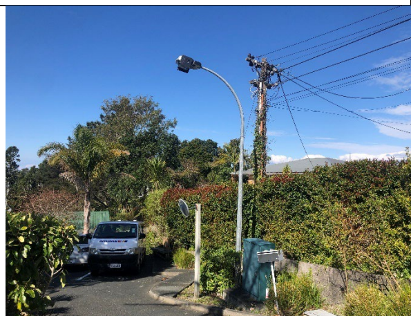
STREETLIGHT TO SECTION AND LAMP TO BE REPLACED. MIRROR BASEPLATE TO BE REPAIRED AND REFIXED IN PLACE.
