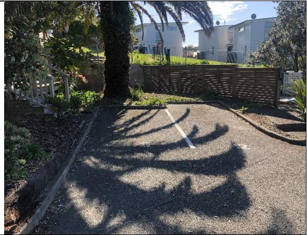
DAMAGED KERBING, AU-53, AU-54.
