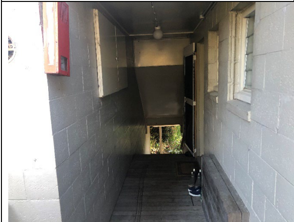
EXAMPLE OF ELECTRICAL BOARDS.
