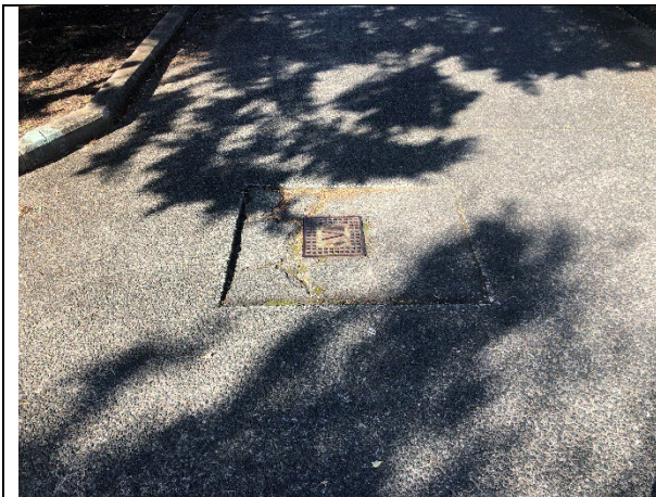
CRACKED AND SUNKEN CONCRETE SURROUND TO WATER SLUICE VALVE TO BE REPLACED ADJ. PU-23
