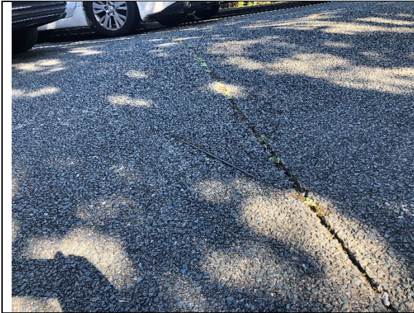
REINFORCING MESH SHOWING AT SURFACE OF CONCRETE, PU-11
