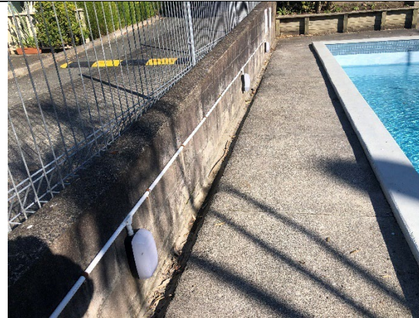
POOL-SIDE LIGHTS NEED REPLACEMENT (FULL OF WATER).
