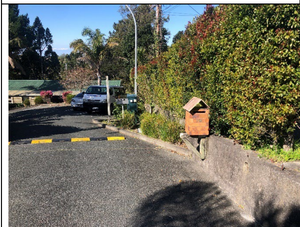
SPEED-BUMB END CAP TO BE REPLACED
