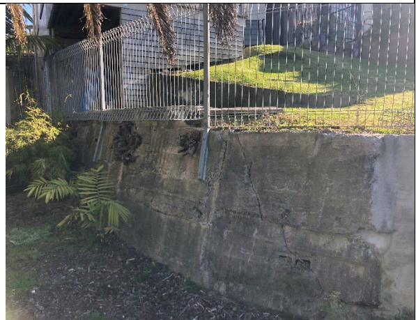
CRACKED RETAINING WALL, PU-7
