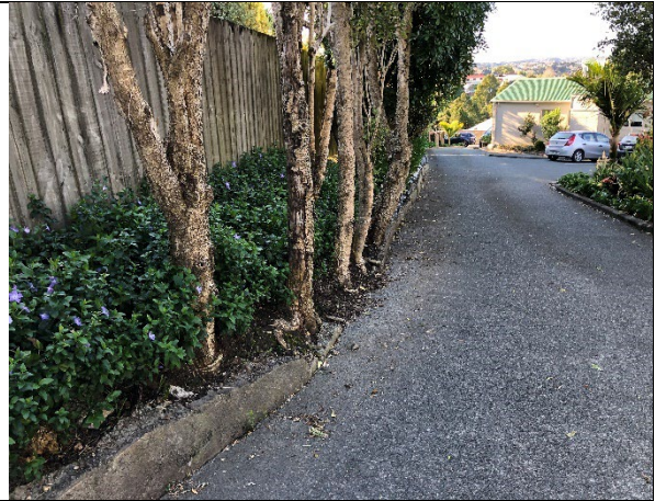
EXAMPLE OF EXCESSIVE SIZED PLANTING WITHIN CONFINED PLANTER. REMOVE TREES AND MAKE GOOD KERBING
