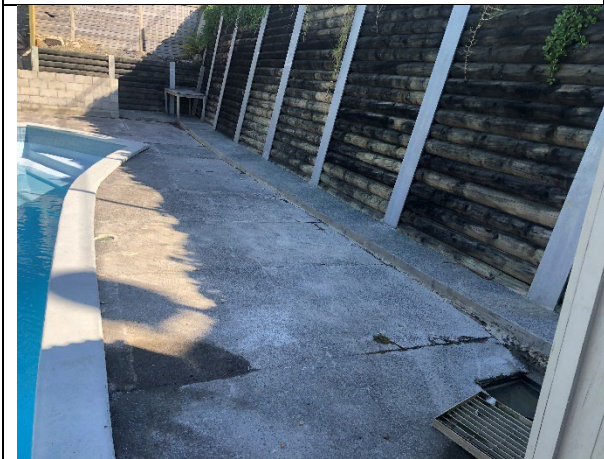
POO-SIDE PATIO CONCRETE NEEDS REPLACEMENT SURFACE WATER SUMP NEEDS UNBLOCKING
