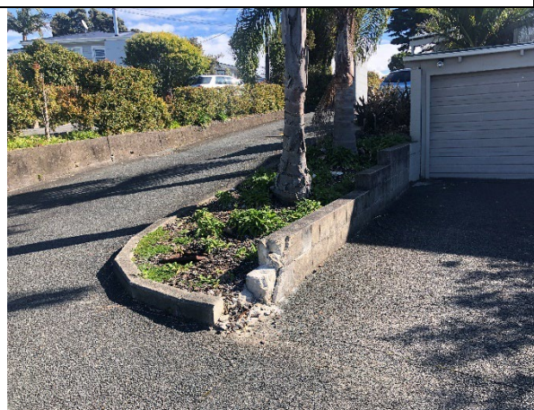
DAMAGED BLOCK WALL AND KERB, PU-23 GARAGE
