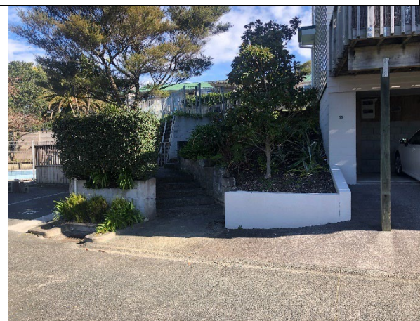
EXAMPLE OF EXCESSIVE SIZED TREE SPECIMEN WITHIN BLOCK PLANTER. TREE ROOTS ARE PUSHING BLOCK WALL OUTWARD. TREE TO BE REMOVED AND WALL REPAIRED, PU-13 & POOL.
