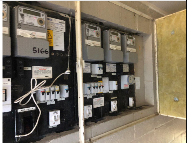
EXAMPLE OF ELECTRICAL BOARDS.
