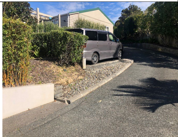
DAMAGED KERBING AU-37, PU-2.
