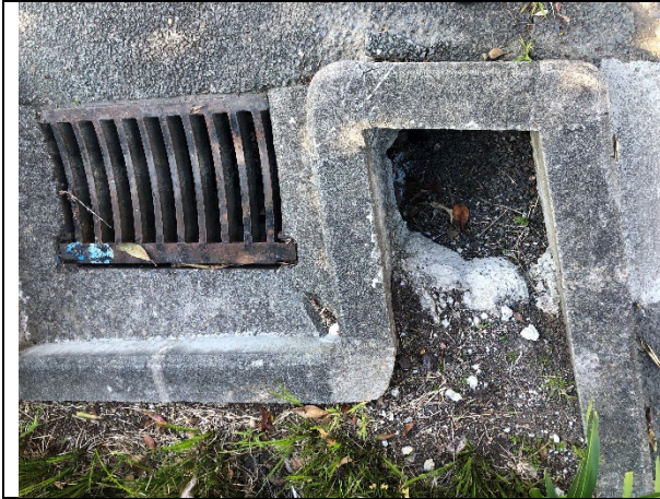
NOVACOIL DRAIN ENTERING SIDE OF CESS PIT REQUIRED REPAIR, PU-13 & POOL.
