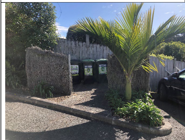
BRUSH-STICK FENCING AROUND RUBBISH AREA TO BE REPLACED, AU-38.
