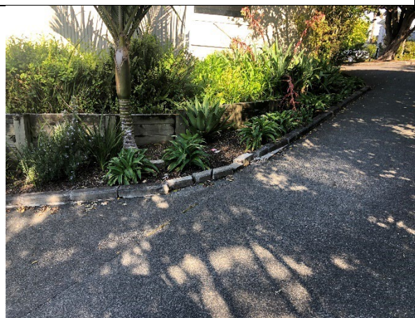
DAMAGED KERBING NORTH-WEST SIDE OF PU-23
