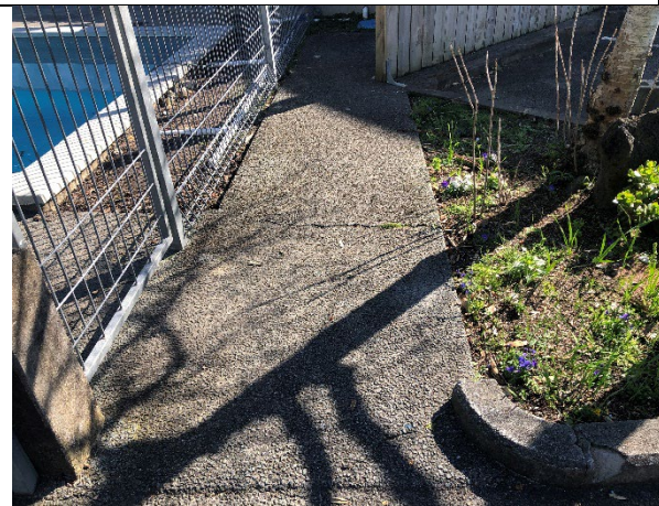
POOL PATH CRACKED
