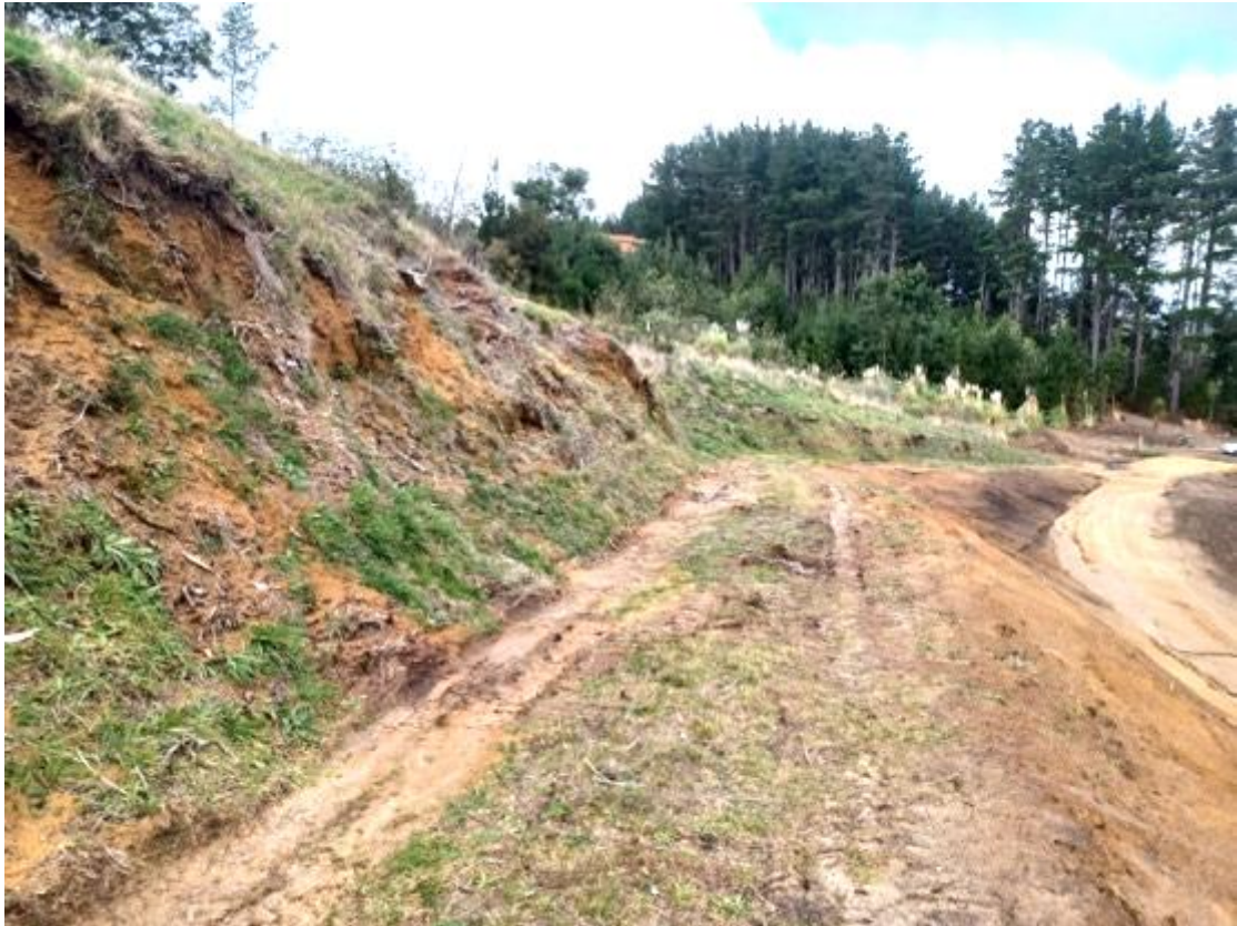
Figure 5: View of the shallow slip on the western slope
