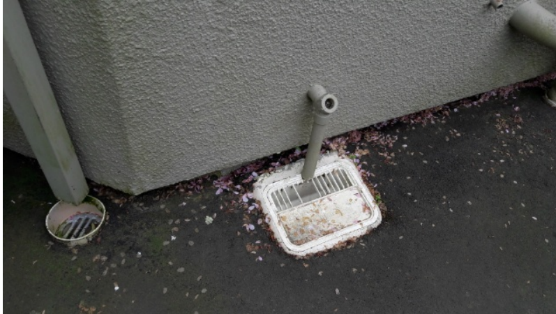
Figure 7 : Services- Gully trap/waste pipe - area of concern raised by the insured. This is not EQ related as the gully trap has pulled away from the foundation over time as evidenced by the historical and discoloured gap between the asphalt surrounding the gully trap and the foundation. The nearby stream would be a contributing factor causing gradule settlement over time. Stream is approximately 5-6 metres away.
