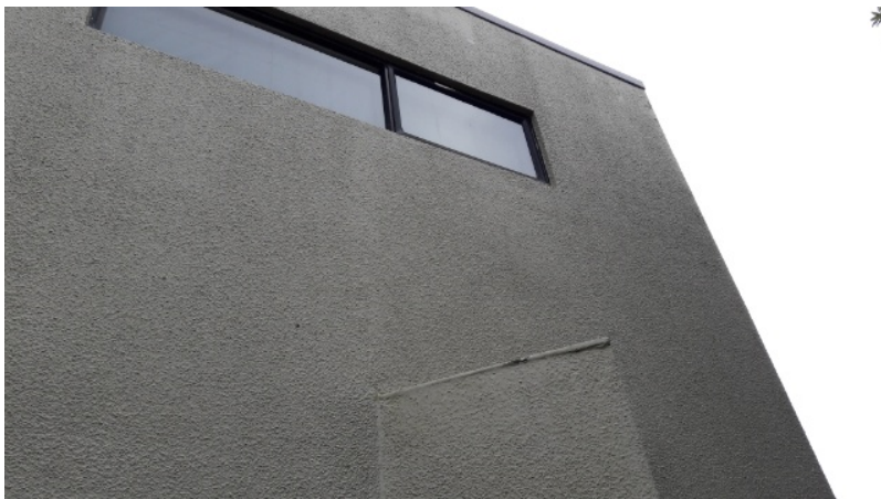
Figure 9 : Plaster render of what appears to be hardie backer rather than Poly. No visible EQ damage.
