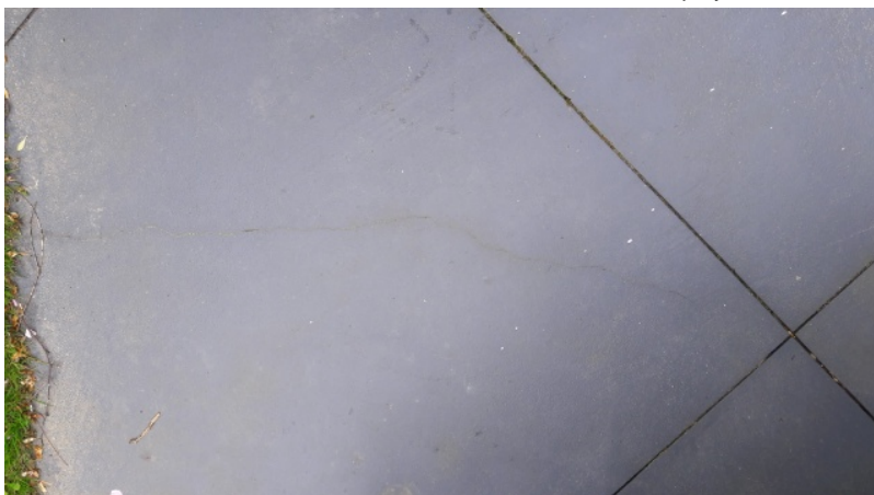
Figure 12 : Insureds partner 'Tom' advised of area of concern to crack in patio. This is not EQ related as evidenced by the rounded edges and debris in the crack. this crack has also been sealed over and displays no fresh related EQ damage.
