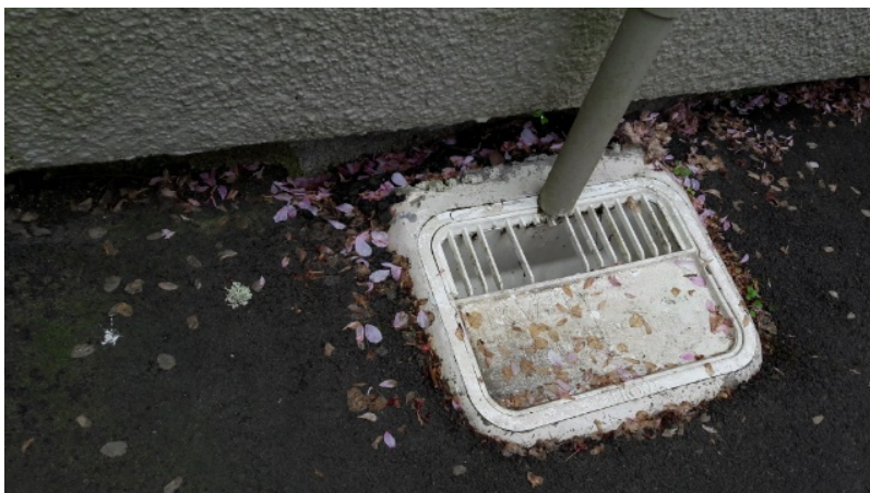
Figure 8 : Services- Gully trap/waste pipe - area of concern raised by the insured. This is not EQ related as the gully trap has pulled away from the foundation over time as evidenced by the historical and discoloured gap between the asphalt surrounding the gully trap and the foundation. The nearby stream would be a contributing factor causing gradule settlement over time. Stream is approximately 5-6 metres away.
