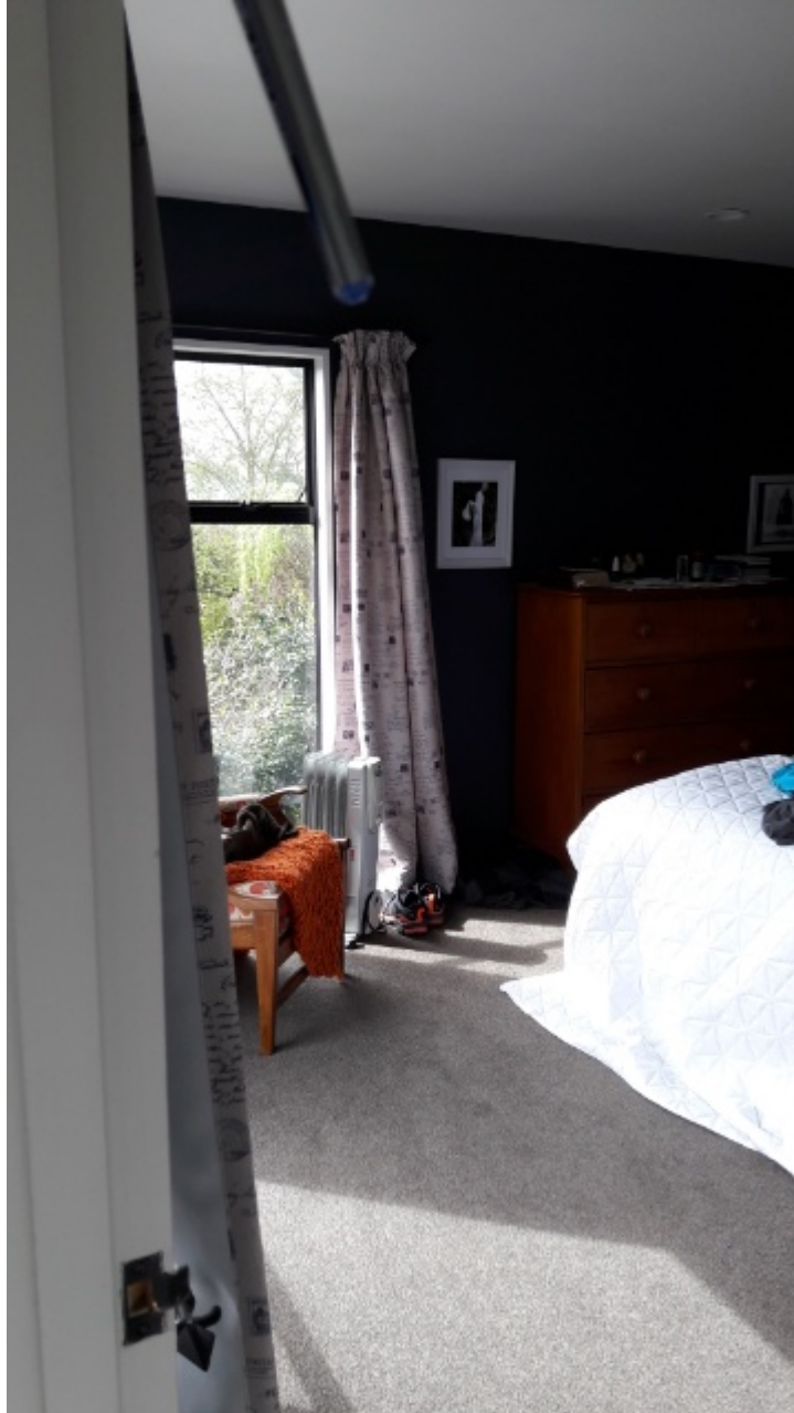
Figure 17 : Bedroom 1 -(2) fresh cracking to wall linings
