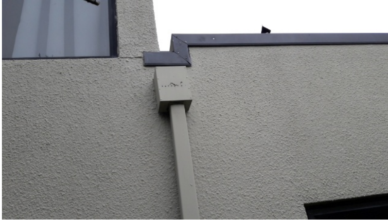
Figure 10 : Plaster render of what appears to be hardie backer rather than Poly. No visible EQ damage.
