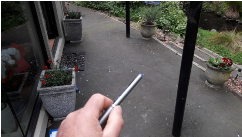
Figure 5 : Asphalt drive- area of concern raised by the insured. These are not EQ related. refer to report notes.
