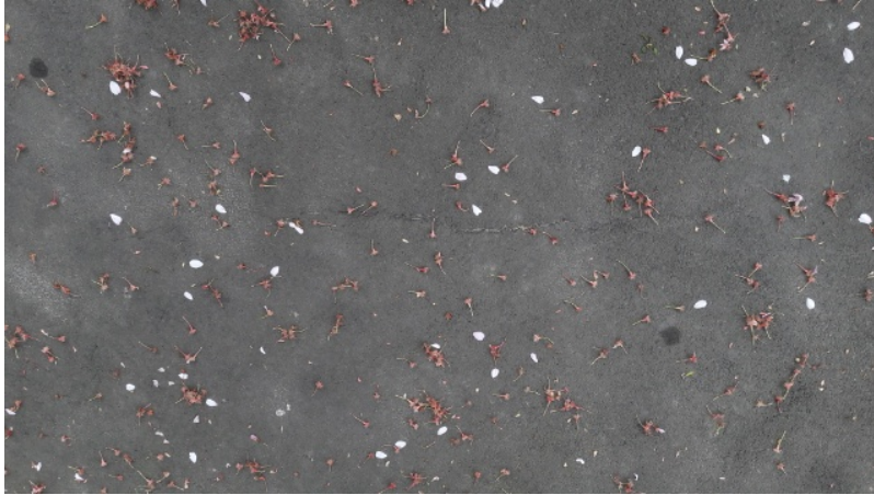
Figure 4 : Asphalt drive- area of concern raised by the insured. These are not EQ related. refer to report notes.
