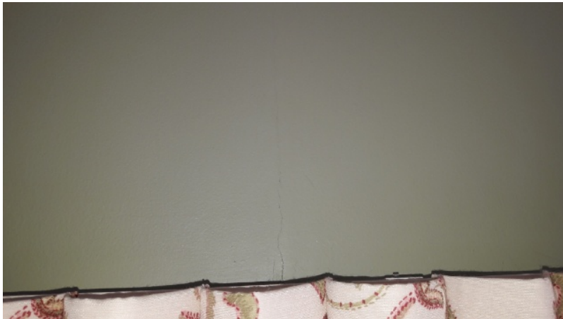
Figure 19 : Bedroom 2 -(1) fresh cracking to wall linings
