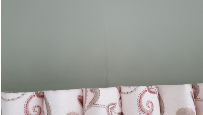
Figure 16 : Bedroom 2 -(1) fresh cracking to wall linings
