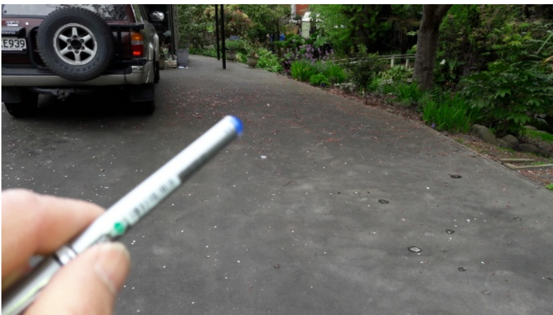
Figure 3 : Asphalt drive- area of concern raised by the insured. These are not EQ related. refer to report notes.
