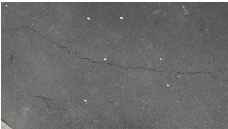
Figure 6 : Asphalt drive- area of concern raised by the insured. These are not EQ related. refer to report notes.
