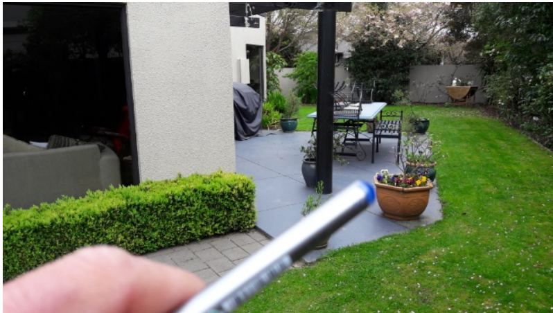
Figure 11 : Insureds partner 'Tom' advised of area of concern to crack in patio. This is not EQ related as evidenced by the rounded edges and debris in the crack. this crack has also been sealed over and displays no fresh related EQ damage.
