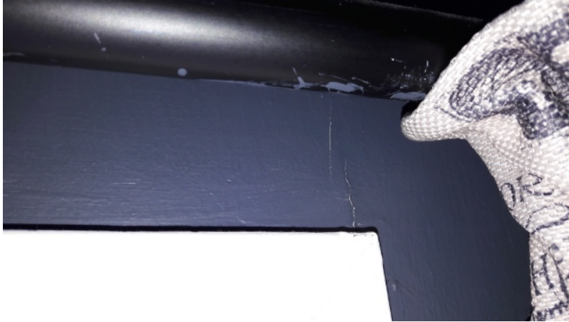
Figure 18 : Bedroom 1 -(2) fresh cracking to wall linings
