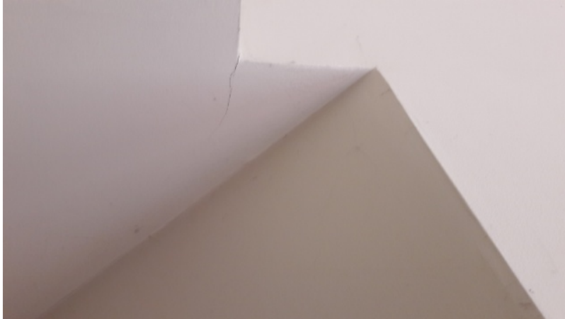
Figure 13 : Front entry- old dark crack observed. Not from this event.
