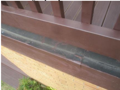
No flashing to parapets
