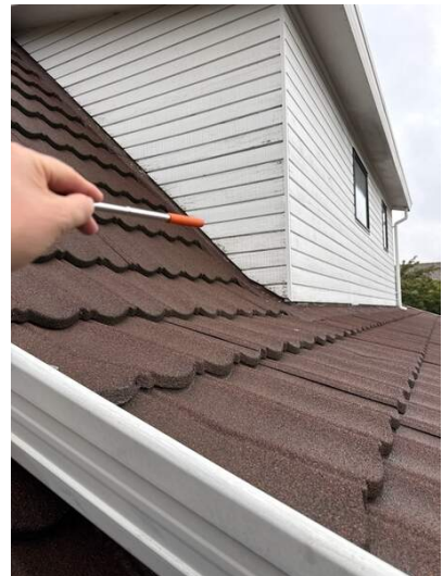
#71: Minor paint deterioration - Eastern elevation
