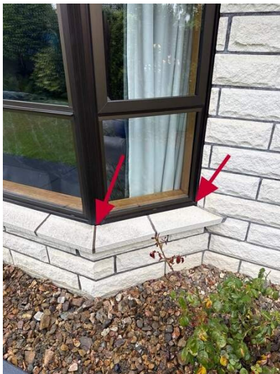
#73: Gaps to mortar - Western elevation
