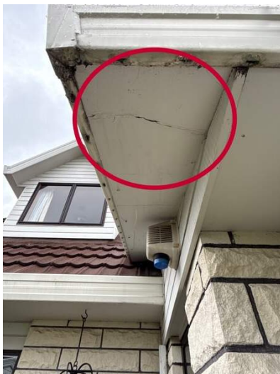
#113: Elevated moisture location - Western elevation
