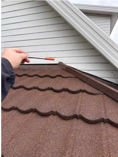
#72: Minor timber split - Southern elevation
