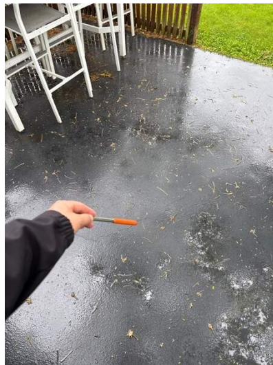
#81: Cracking to concrete
