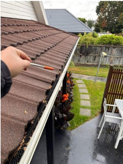
#99: Popped nails - Southern elevation
