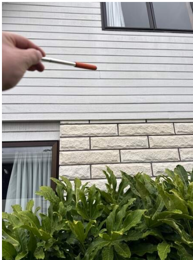
#69: Weatherboard joints opening up - Northern elevation
