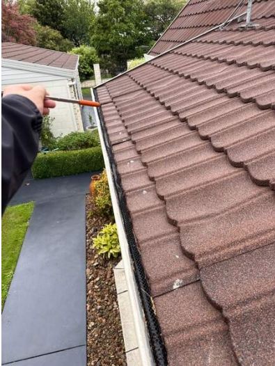
#96: Popped nails - Western elevation
