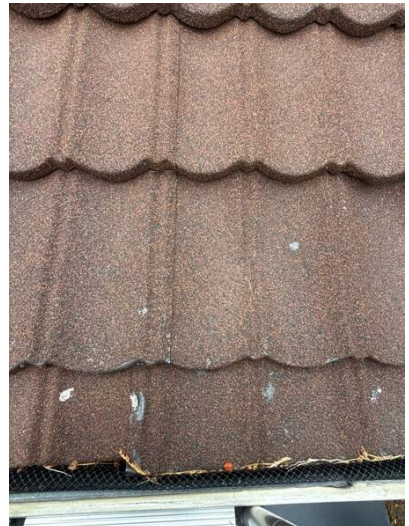
#101: Minor coating deterioration
