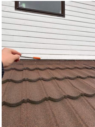
#70: Minor paint deterioration - Eastern elevation
