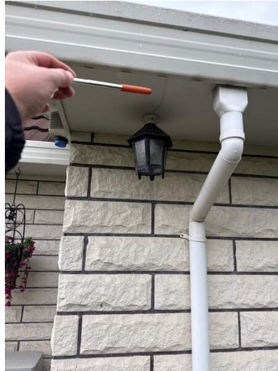
#105: Cracked eave lining - Western elevation
