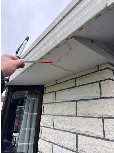
#104: Cracked eave lining - Western elevation
