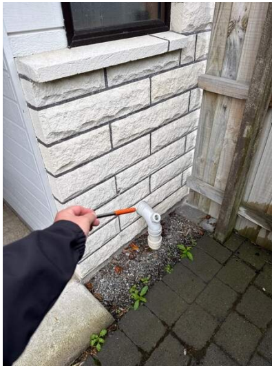
#75: Unsealed cladding penetrations - Eastern elevation
