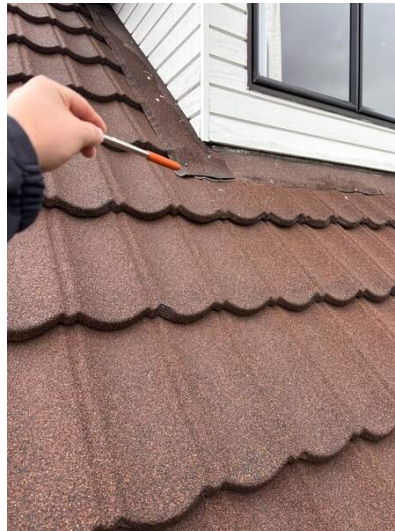
#94: Popped nail - Western elevation
