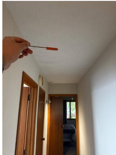
#137: Smoke alarm required - First-floor hallway
