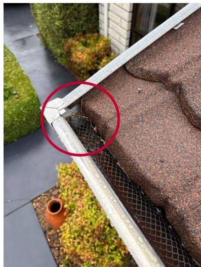
#114: Gaps at barge flashing junction - Western elevation
