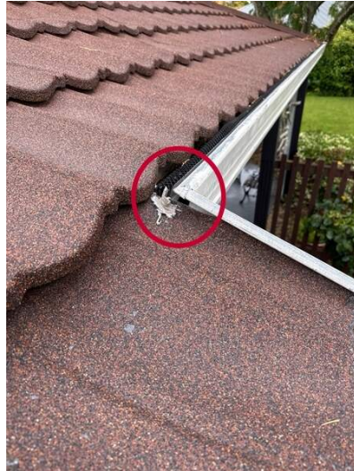
#117: Gaps at fascia - Western elevation
