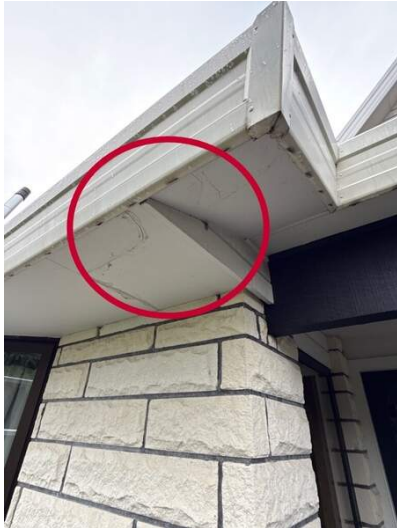
#116: Elevated moisture location - Western elevation
