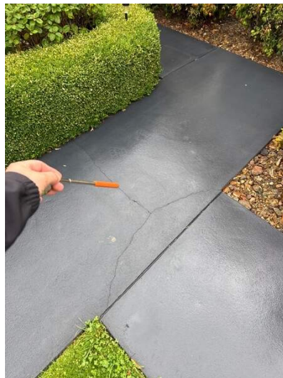
#156: Cracking to concrete
