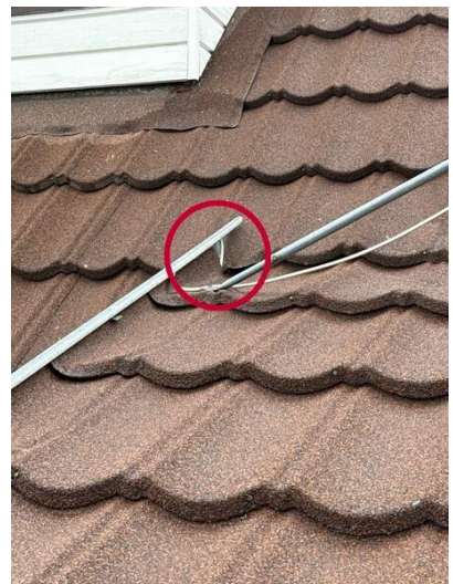
#115: Gaps at barge flashing junction - Western elevation
