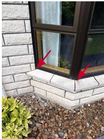
#74: Gaps to mortar - Western elevation
