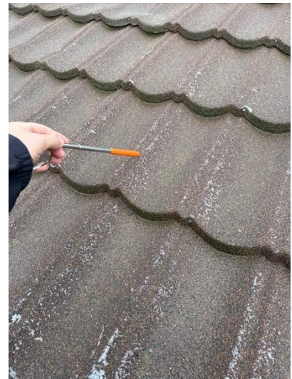
#148: Minor coating deterioration
