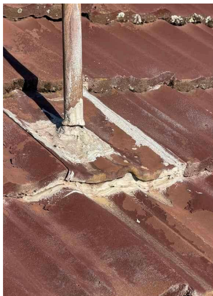
previous repairs noted to vent.
