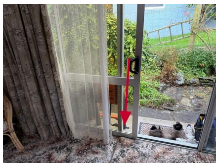
#29: Rollers require maintenance.
