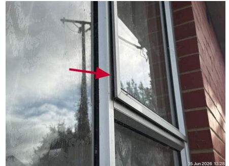
#92: Gaps around the closed sash
