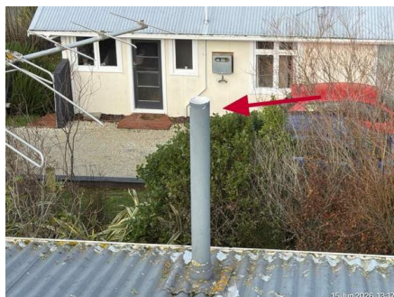
#204: No vermin cap to the vent.
