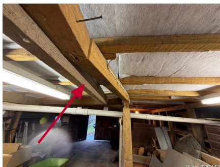
#168: Modifications and poorly supported bearers.
