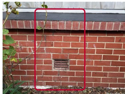
#78: Cracking western face.
