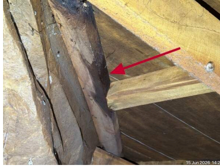
#139: Moisture staining to the framing visible.
