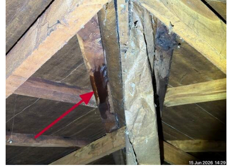
#140: Moisture staining to the framing visible.
