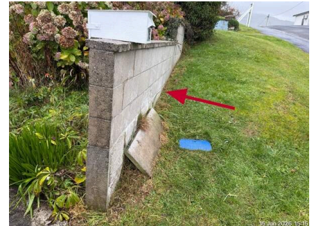
#241: Front masonry fence is on a lean.
