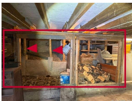
#171: Modifications and poorly supported bearers.
