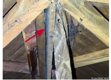
#147: Sagging paper and gaps visible.
