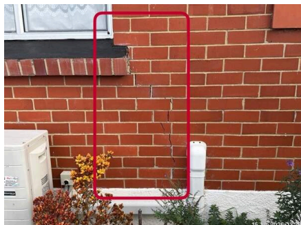
#76: Cracking to the northern face.
