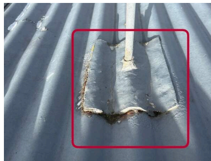
#120: Older flashing with corrosion and gaps present.
