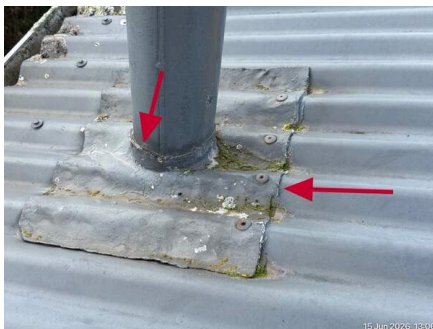
#119: Older penetration flashing showing signs of deterioration. And gaps around the pipe junction.
