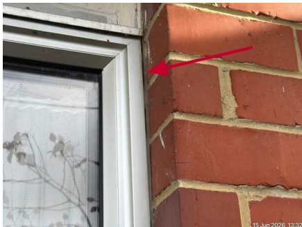
#93: Gaps in the sealant around the windows.
