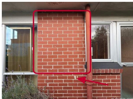
#79: Cracking and newer bricks in place indicating previous repairs.
