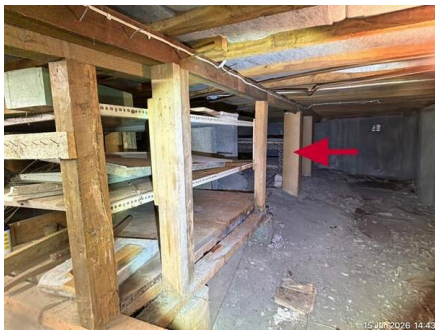
#159: Leaning piles visible.
