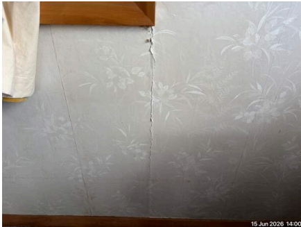
#18: Cracking visible in multiple locations.
