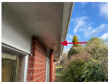
#128: Moisture staining and sagging visible to the eave linings.
