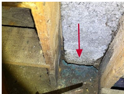
#163: Settlement noted to the northern and eastern sections of the foundation.
