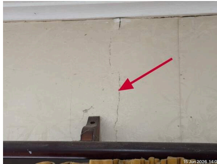
#19: Cracking visible in multiple locations.
