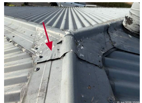
#114: Older hip cap with multiple old penetration holes visible.
