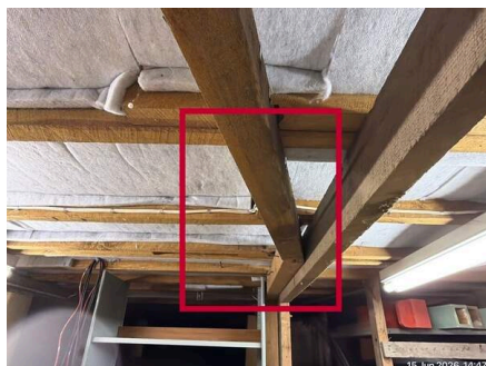
#167: Modifications and poorly supported bearers.
