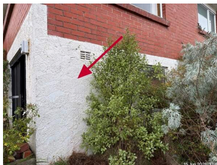
#88: General paint deterioration.
