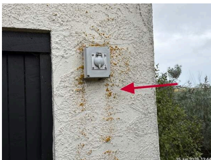
#87: Moss and lichen growth to the foundation paint in various locations around the dwelling.
