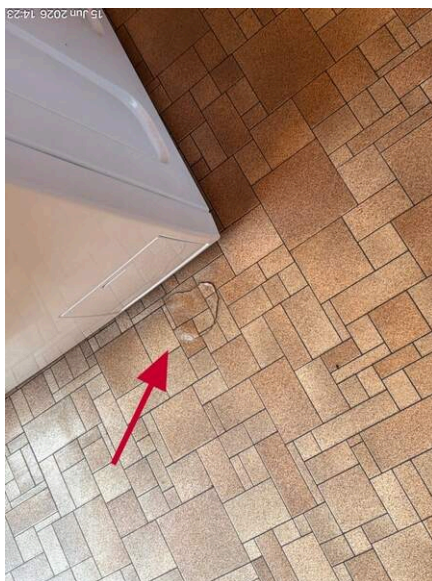
#65: Tear to the flooring.
