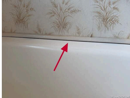
#50: Gaps to the bath trim junction.
