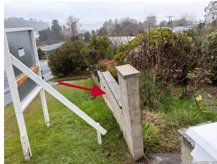
#240: Front masonry fence is on a lean.
