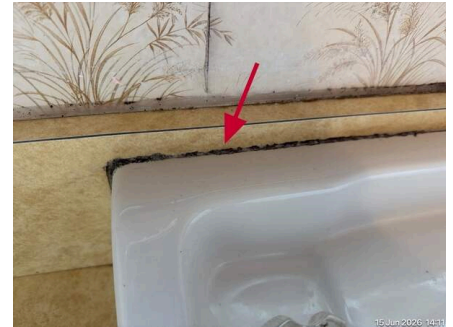
#58: Mouldy deterioration to the sealant.
