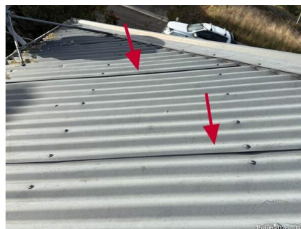
#113: Sheet edge lifting visible.
