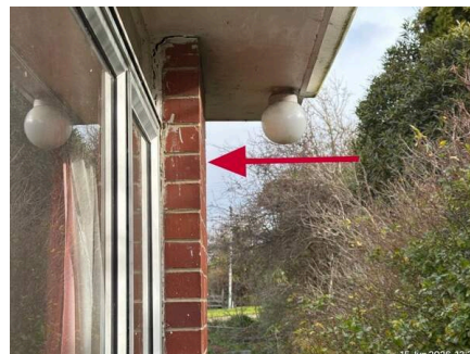
#81: Vertical movement to the brickwork visible at the SW corner.
