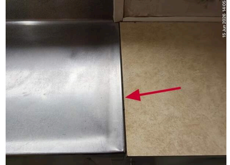
#33: Gaps at the benchtop junction.
