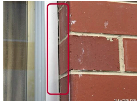
#95: Gaps at the joinery to cladding junction.
