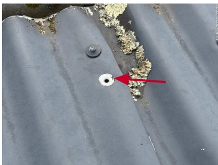
#112: Unsealed fixing penetrations in various locations.
