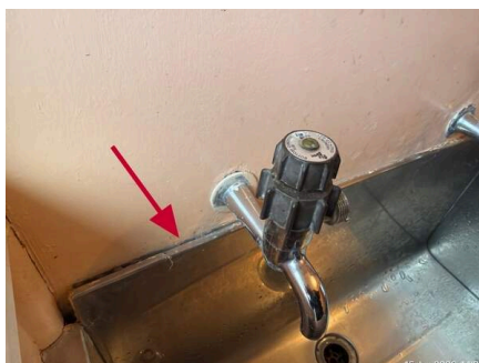
#63: Tub is not sealed to the wall.
