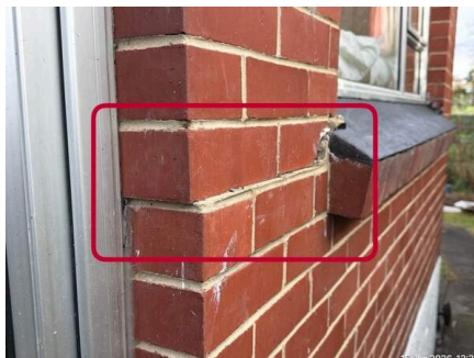
#80: Extensive movement visible to the western face.
