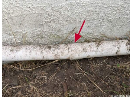
#207: Loose downpipe join.
