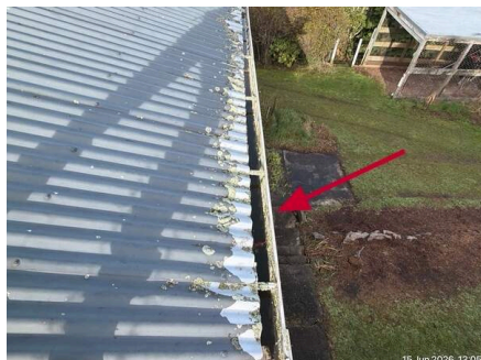
#124: South facing gutter is holding water.
