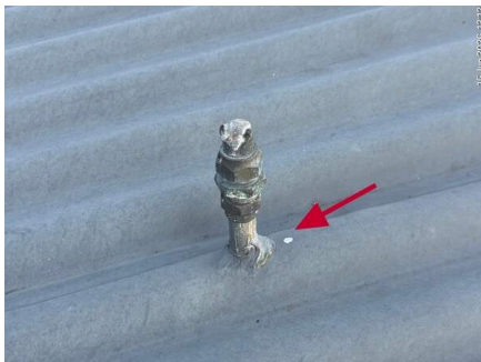
#122: Poorly sealed penetration.
