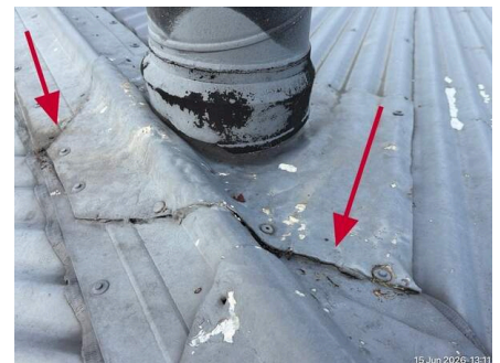
#121: Older flue penetration flashing with gaps visible and flashing corrosion visible.
