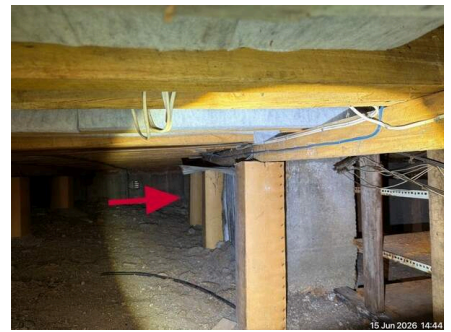
#161: Leaning piles visible.
