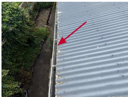
#125: West facing gutter is holding water.
