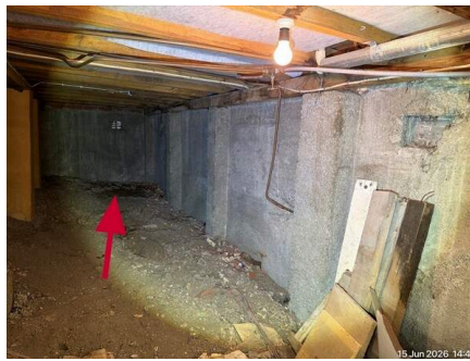
#160: Settlement noted to the northern and eastern sections of the foundation
