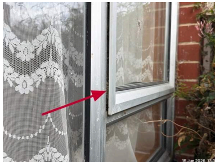
#94: Gaps around the sashes.
