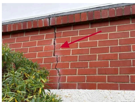
#82: Extensive crack to the south face.
