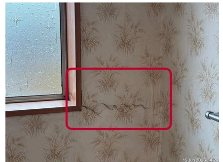
#23: Cracking to the bathroom linings.
