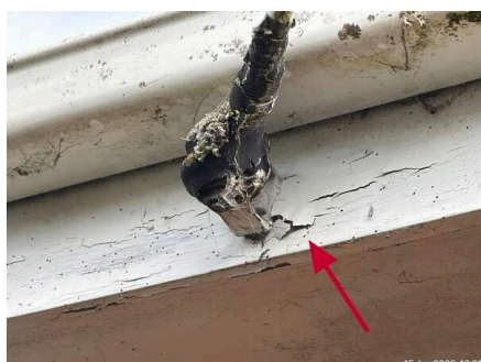
#130: Borer and paint deterioration.
