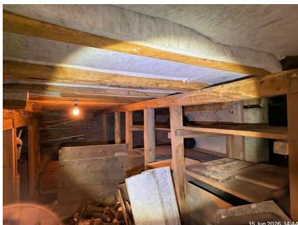
#162: Leaning piles visible.
