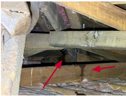
#141: Moisture staining to the framing visible.
