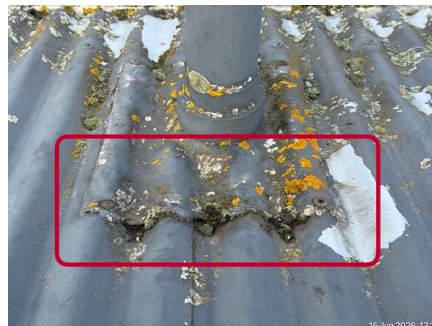
#123: Corrosion and gaps at the flashing junction.
