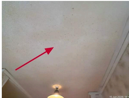
#17: Paint deterioration and staining to the bathroom ceiling.
