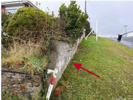
#239: Front masonry fence is on a lean.
