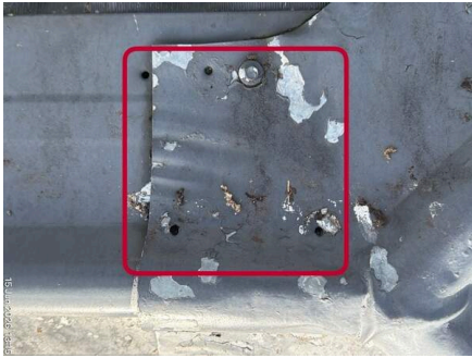
#118: Multiple unsealed penetration holes.
