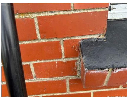
#83: Cracking and lateral movement visible to the SE corner.
