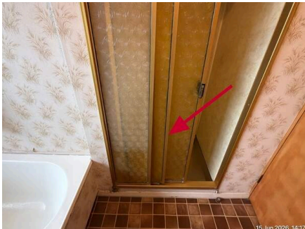
#52: Shower doors are broken.
