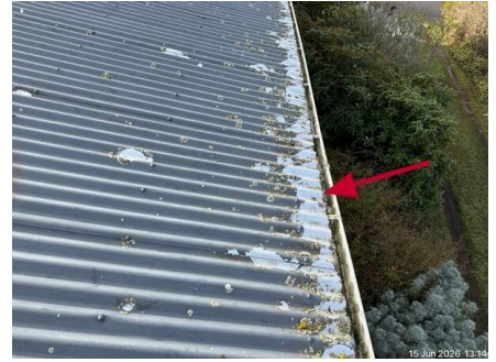
#117: Extensive sheet edge deterioration.
