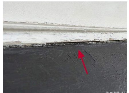
#98: Gaps to the sill south face.
