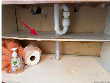
#57: Moisture damage from the waste leak.
