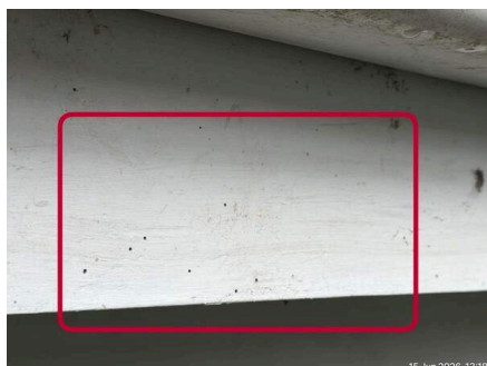
#127: Borer holes in the Fascia.
