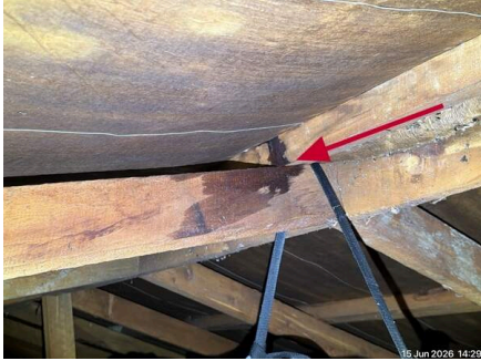
#138: Moisture staining to the framing visible.
