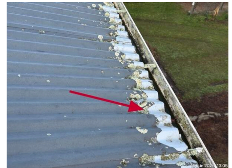
#111: Coating delamination due to moss and lichen.
