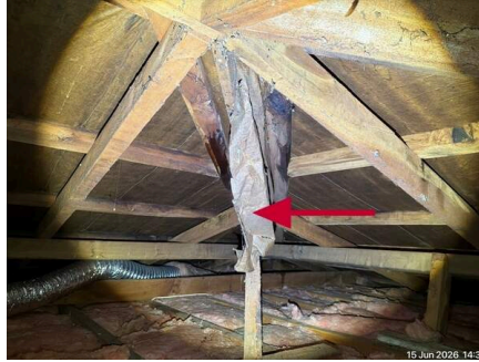
#146: Sagging paper and gaps visible.
