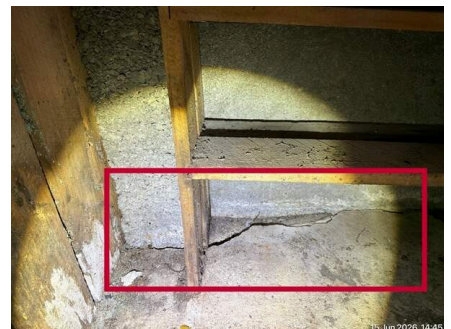
#164: Settlement noted to the northern and eastern sections of the foundation.
