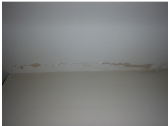
Photo 3 – Damage to plaster at corner joints between plasterboard elements
