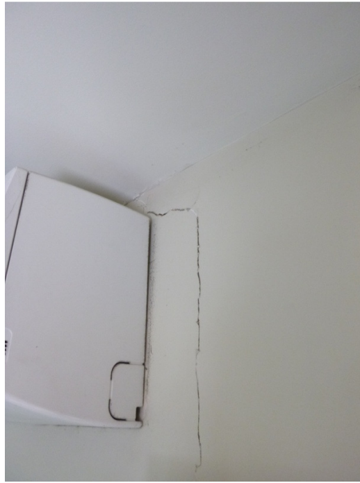
Photo 2 – Plasterboard element to be replaced
