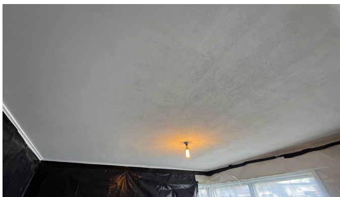
Stage 2 - Textured coating removed from bedroom ceiling
