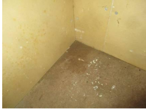
Minor leakage into bay windows (dry reading)
