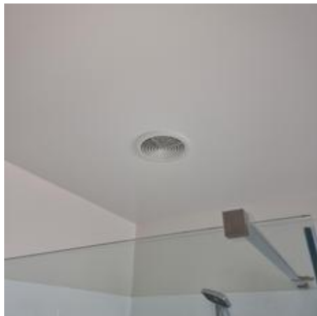
Photo of Extractor fan
