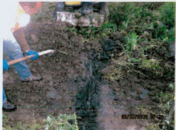
Photo 2. Distribution pipe (40mm) showing gravel pack blocked with black biomat.
