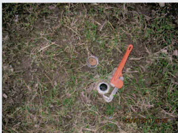
Photo 4. Distribution pipe flush-out port at end of line
