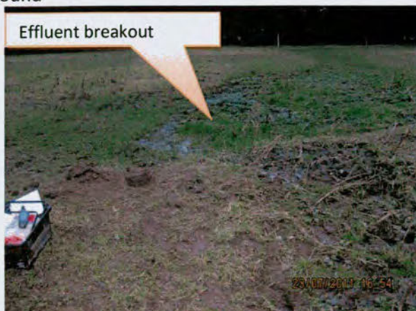
Photo 2 Mound showing effluent breakout at east of mound
