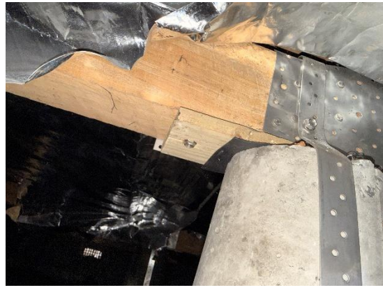
Photo 10. View of internal pile packer.
