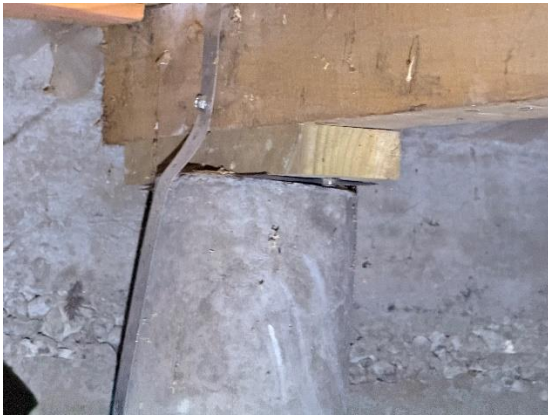
Photo 9. View of internal pile packer.
