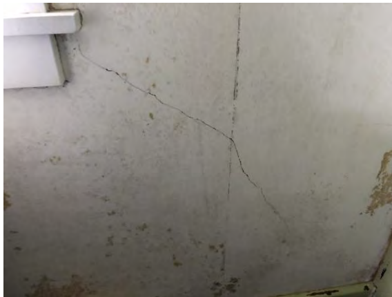
Photo 6. Cracking damage to the plasterboard.
