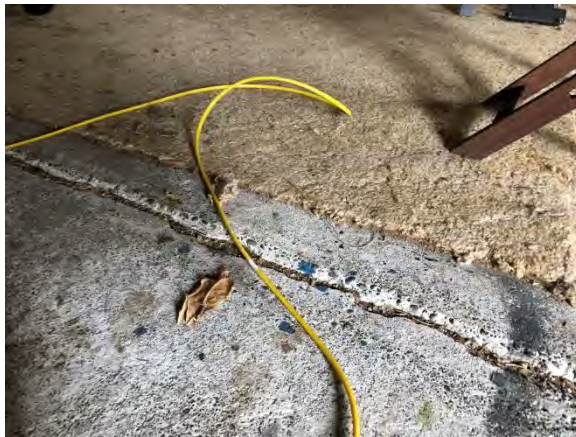
Photo 16. Vertical offset along the construction joint of the garage slab.
