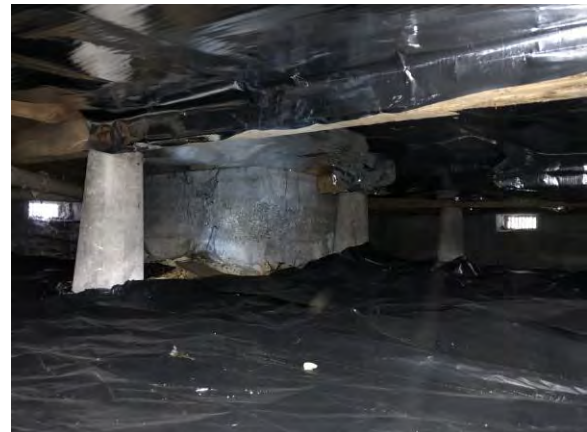
Photo 13. Concrete base observed underneath the sagging floor.
