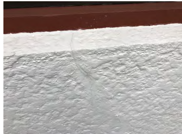
Photo 5. Crack repaired then re-opened.
