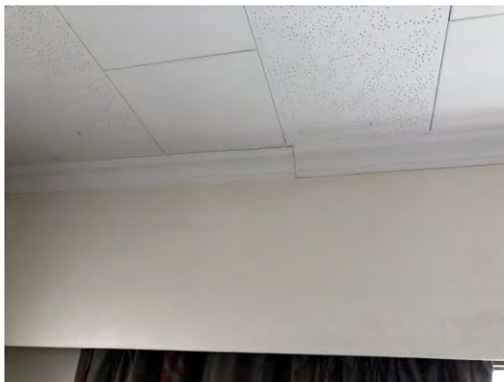
Photo 8. Movement and cracking damage to the scotia.
