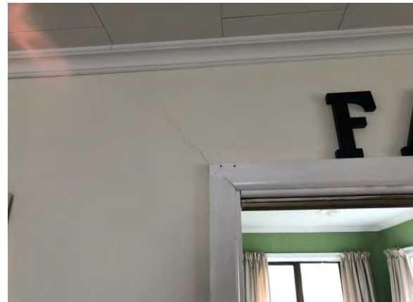
Photo 7. Cracking damage to the wall lining around the door opening.
