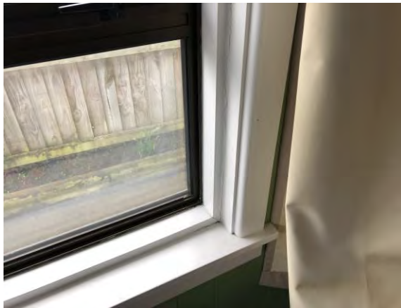
Photo 10. Cracking damage along the window frame.
