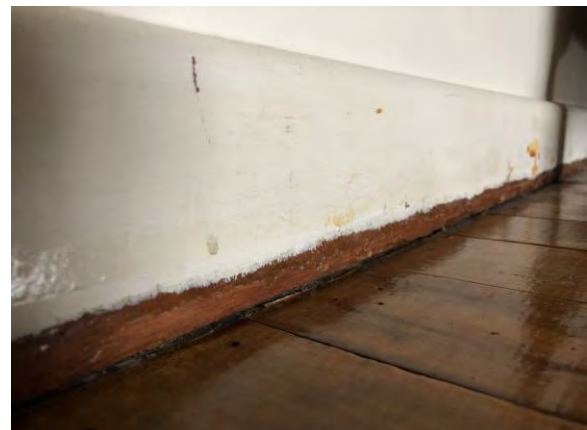
Photo 9. Separation between the skirting board and sagging floor.
