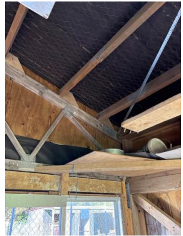
Roof paper overall good.
