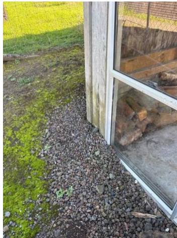
Cladding in contact with ground.
