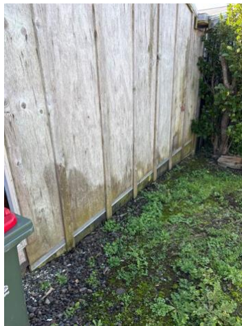
Cladding in contact with ground.
