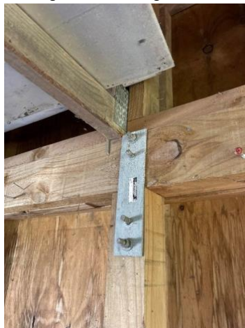
Adequate connections. Some additional bolts required.
