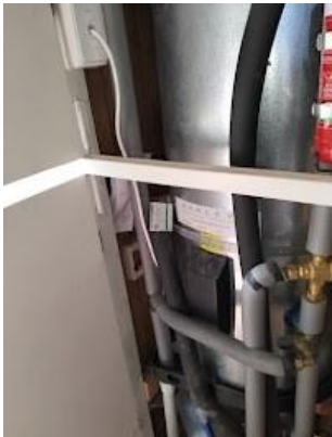
Hot Water Heater
