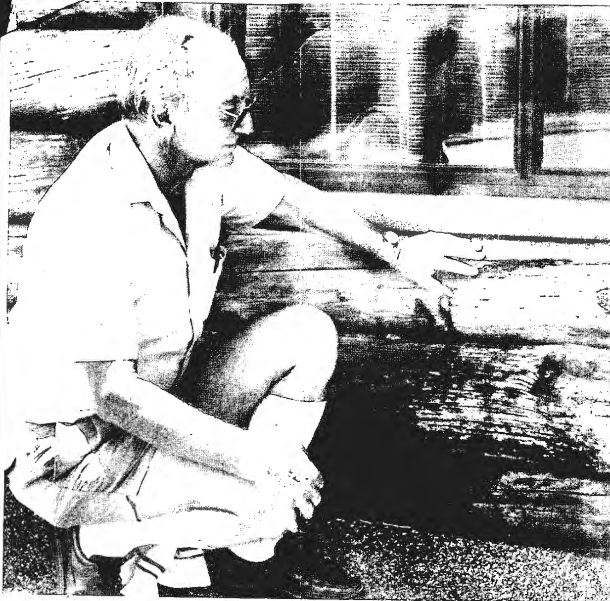
□ Mr Sutherland examines the deterioration of logs in the Kaikohe cabin.
