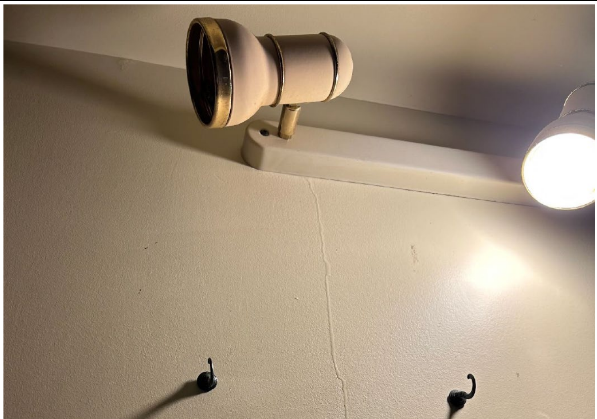
6.15 Image provided by Owner of Unit 28 showing water leak to Level 2 Bedroom wall during Event.
