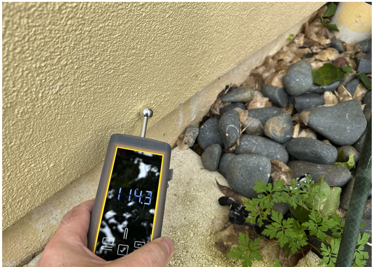
6.6 High moisture reading at cladding base
