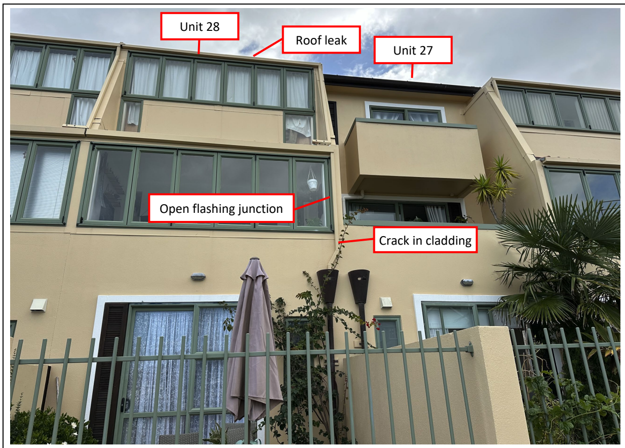
6.1 Overview of the Units with areas of concern arrowed.
