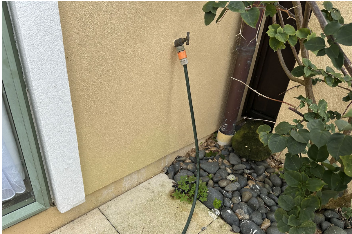
6.5 Cladding beneath bathroom window in Unit 28 showing efflorescence and staining
