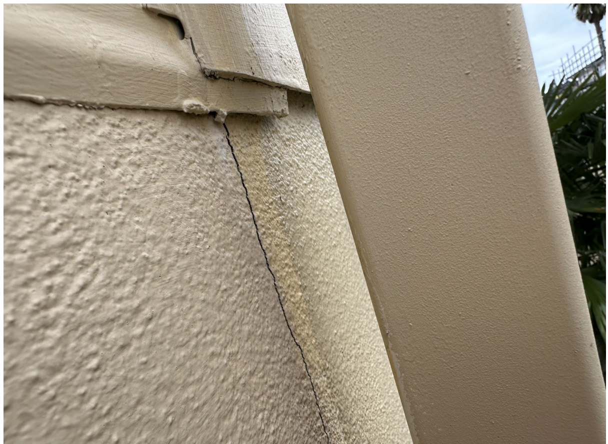
6.3 Cracking in exterior cladding
