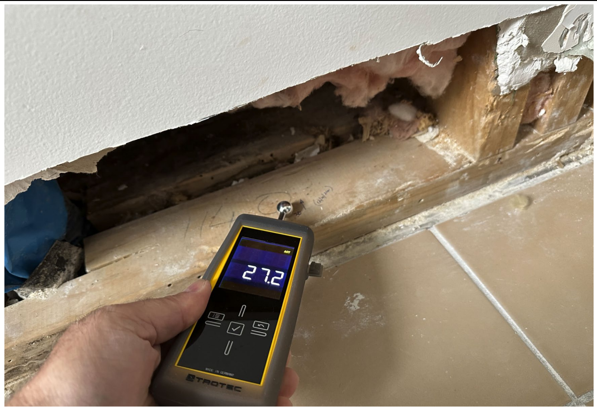
6.9 Slightly elevated moisture content in bottom plate on Unit 27 side of intertenancy wall
