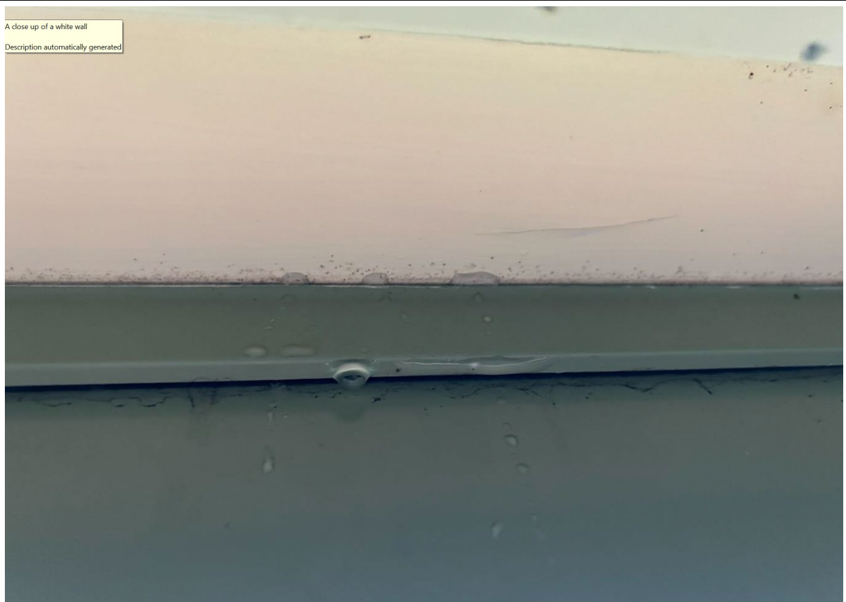
6.16 Image provided by Owner of Unit 28 showing water leak to Level 2 Bedroom joinery during Event
