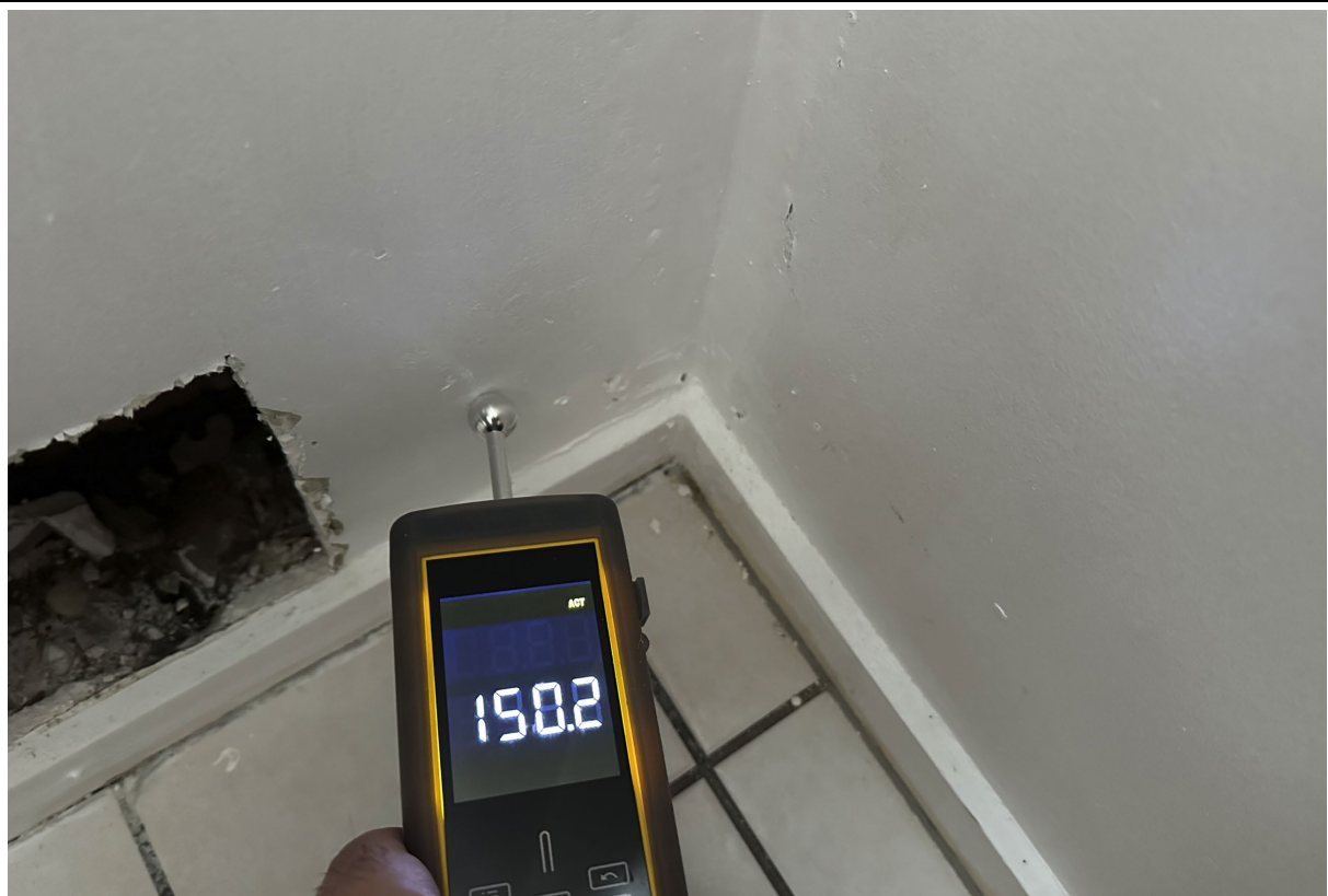
6.19 Highly elevated moisture content reading in external wall of Unit 28 Ground floor Bathroom
