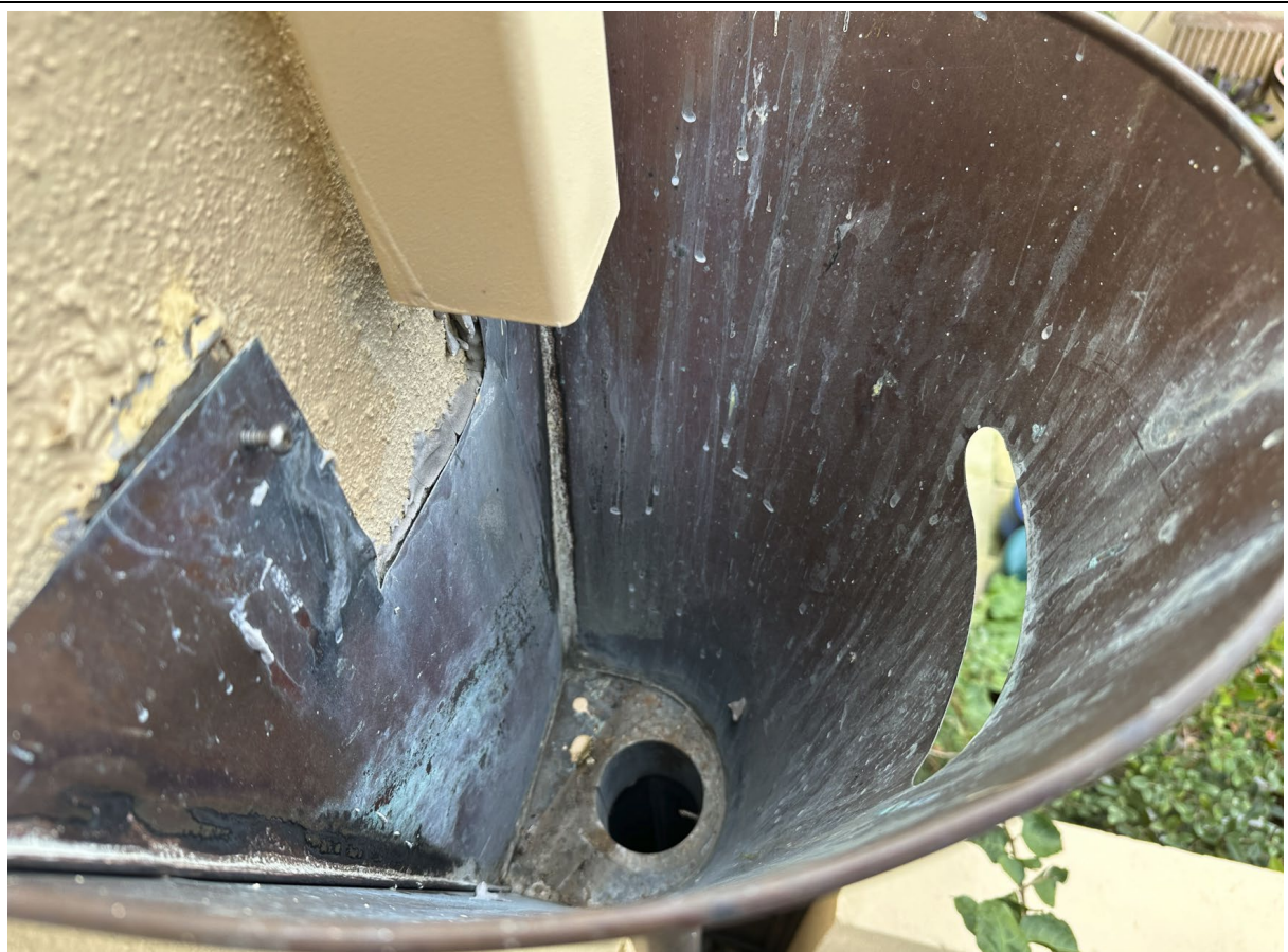
6.4 Poor sealing around rainwater head
