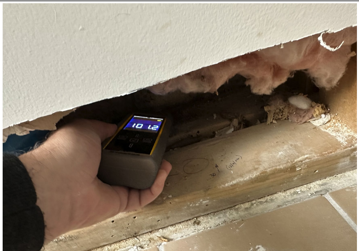
6.10 Highly elevated moisture content in bottom plate on Unit 28 side of intertenancy wall
