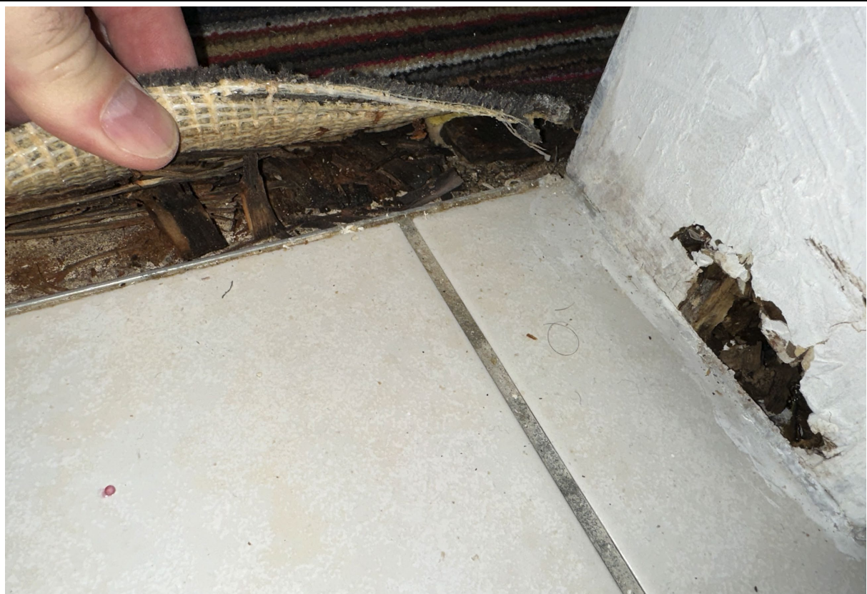
6.20 Timber decay in door reveal and carpet edging near shower end of Unit 28 Ground Floor Bathroom
