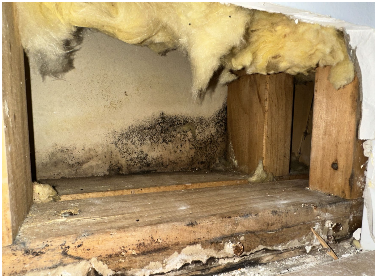
6.11 Fungal growth and timber decay in the bathroom intertenancy wall
