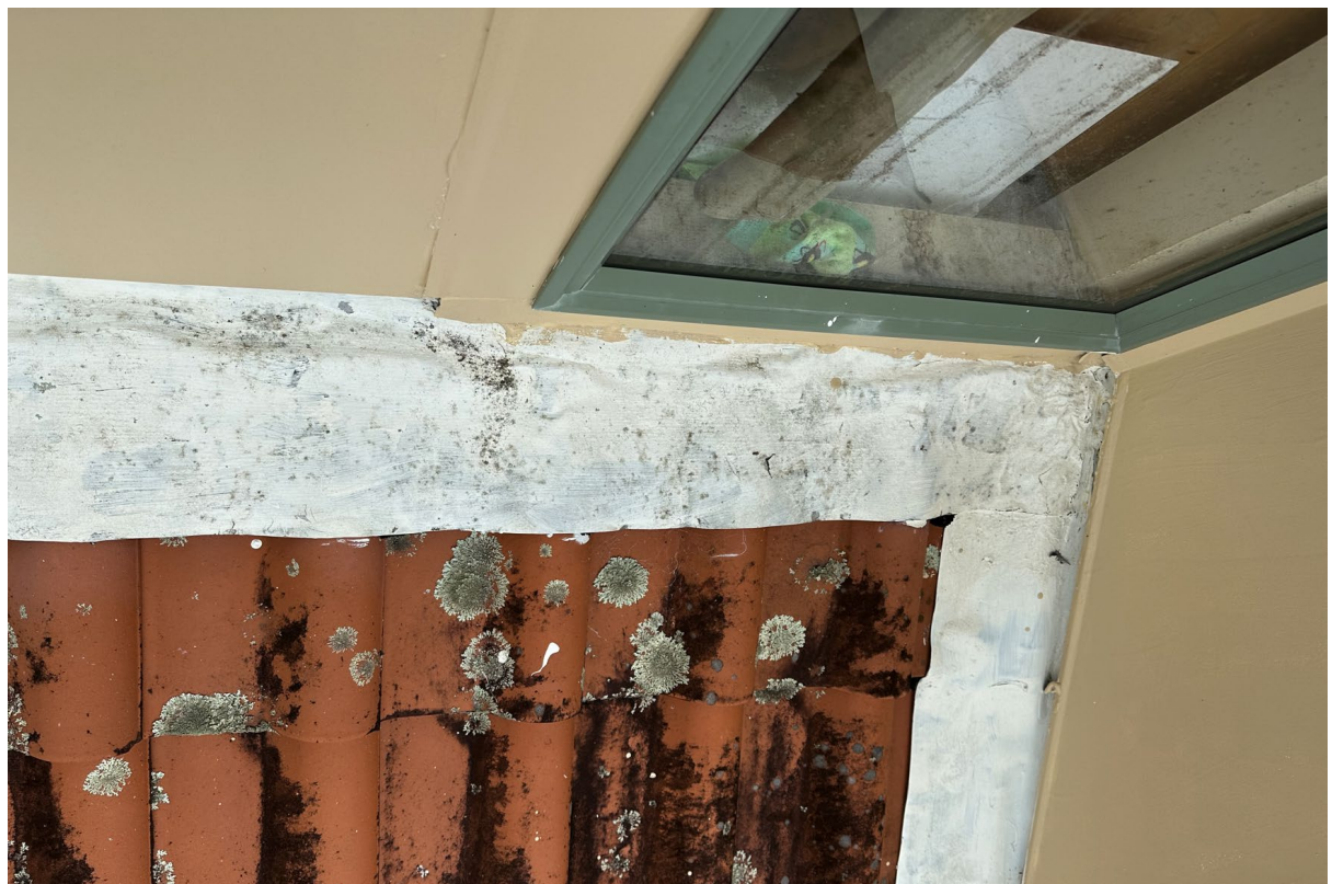
6.14 Moisture damage to window reveals (now dry) as viewed through Level 2 Bedroom window
