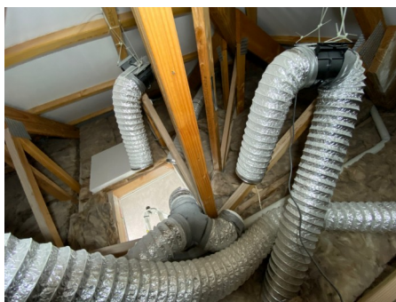
Bathroom 1 extraction system ducting Ducting is disconnected and system vents into ceiling cavity. View High Resolution Image Here
