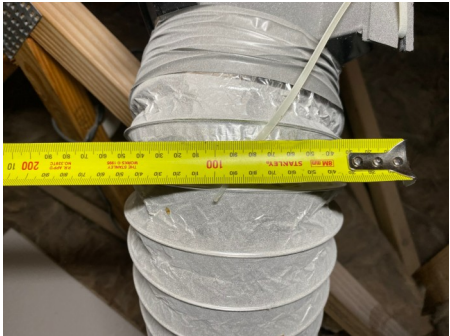
Bathroom 2 extraction system ducting 150mm View High Resolution Image Here
