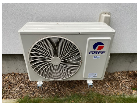
Exterior Heating system/condenser Heat pump, Gree GWH18AGDXE-K6DNA1A/O View High Resolution Image Here
