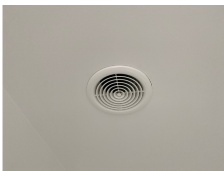
Bathroom 1 extraction system Extraction system vents back into ceiling cavity. View High Resolution Image Here
