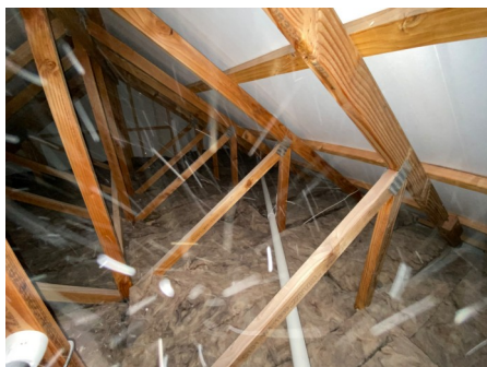
Ceiling Cavity Insulation consists of Fibreglass. View High Resolution Image Here
