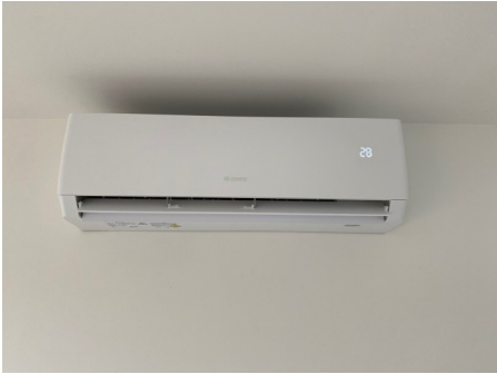
Heater Heat pump, Gree GWH18AGDXE-K6DNA1A/O Good working condition and produces heat. View High Resolution Image Here
