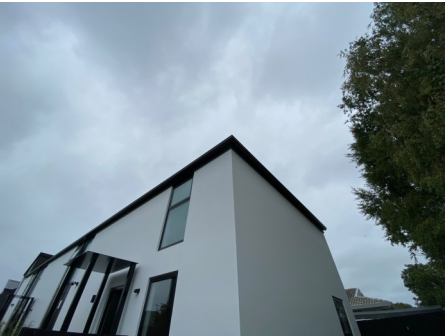
Bathroom 2 extraction system external vent External vent located at the roof. View High Resolution Image Here
