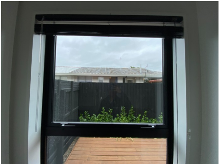
Kitchen The window is compliant for draught stopping. View High Resolution Image Here
