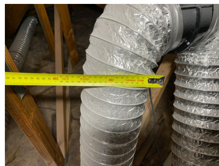
Bathroom 1 extraction system ducting 150mm View High Resolution Image Here
