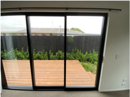
Lounge The door is compliant for draught stopping. View High Resolution Image Here
