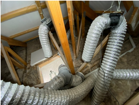
Bathroom 2 extraction system ducting Ducting is disconnected and system vents into ceiling cavity. View High Resolution Image Here
