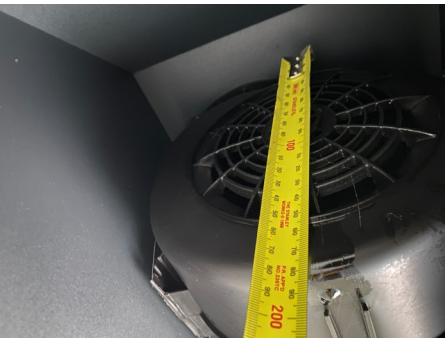
Kitchen extraction system ducting Ducting measurement is 150mm. View High Resolution Image Here
