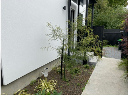
Subfloor surrounds - Front of property There is no sub floor as the property is built on a concrete foundation. View High Resolution Image Here
