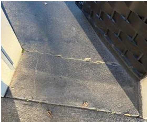
Cracking to paths
