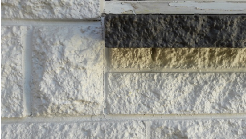
Figure 7 : Cladding damage west side of dwelling.
