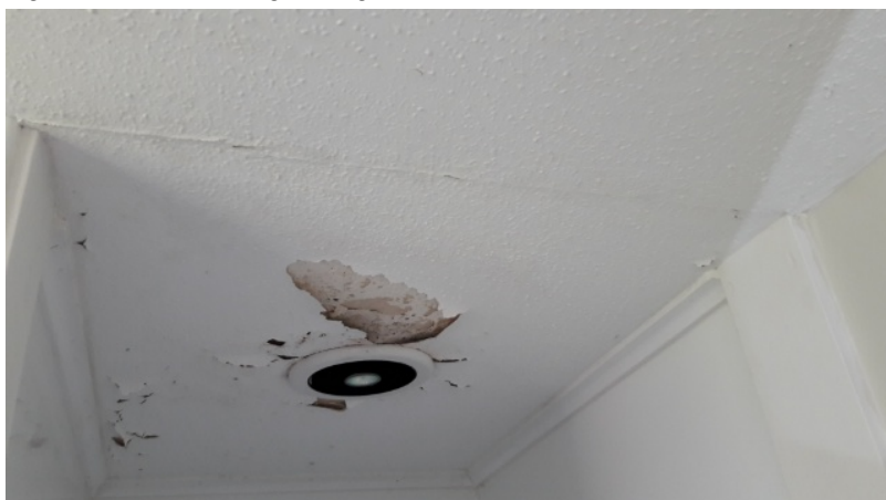
Figure 2 : Historical ceiling damage Bathroom area
