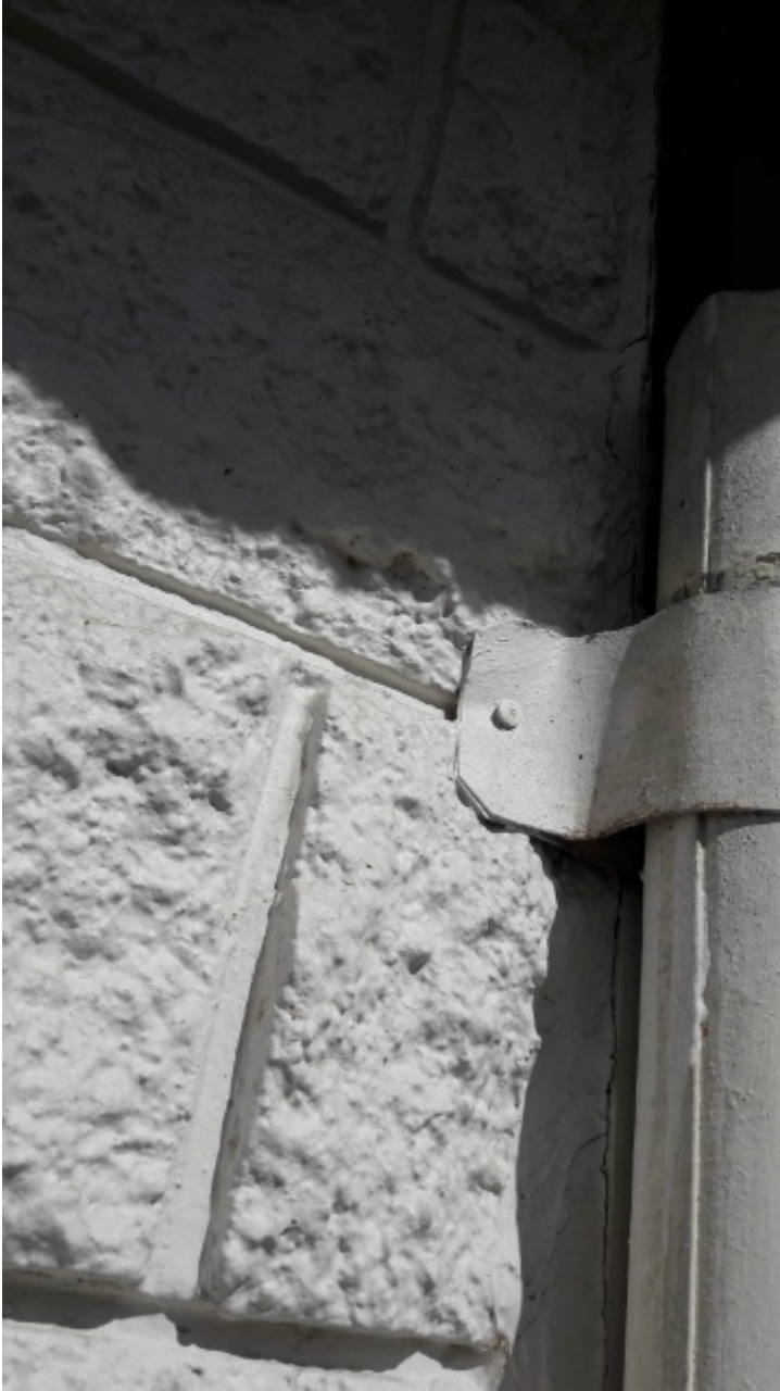
Figure 5 : Cracking between Sunroom and brick veneer, north side of dwelling.
