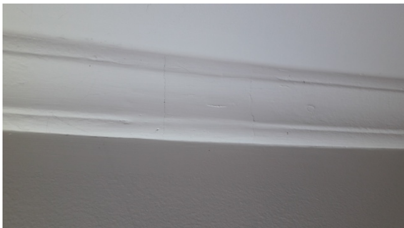
Figure 1 : Cornice damage Lounge area
