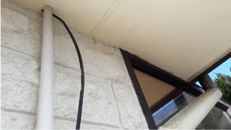
Figure 6 : Cracking between Sunroom and brick veneer, north side of dwelling.
