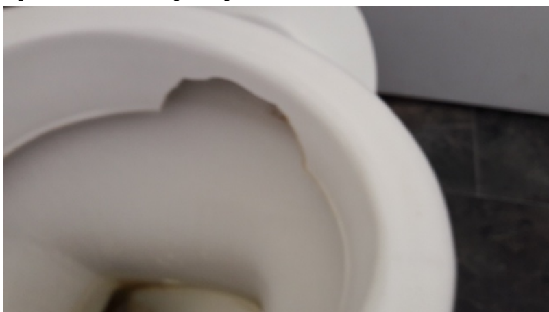
Figure 3 : Pan damage Toilet area
