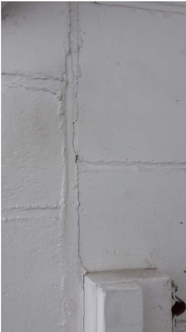
Figure 9 : Mortar line cracking north side of Garage.
