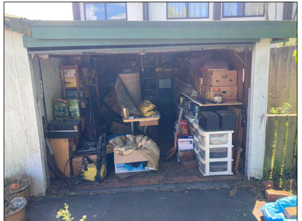
Photo 7B – Garage was full of storage at the time of the assessment. Door head was measured to be level over sloping concrete slab.
