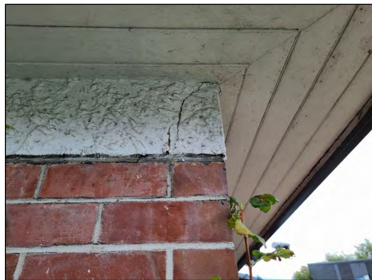
Photo 3F – Separation at the corner joints of the precast concrete beam above the veneer panels at the exterior north east corner of the kitchen.
