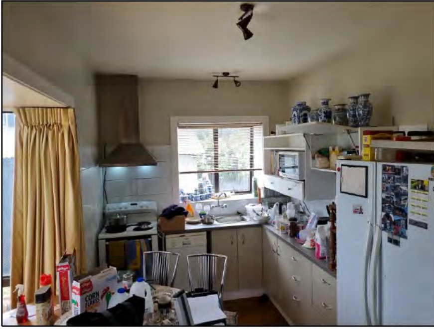
Photo 4A –Kitchen floors , ceilings and built in benchtops all fall to the north.
