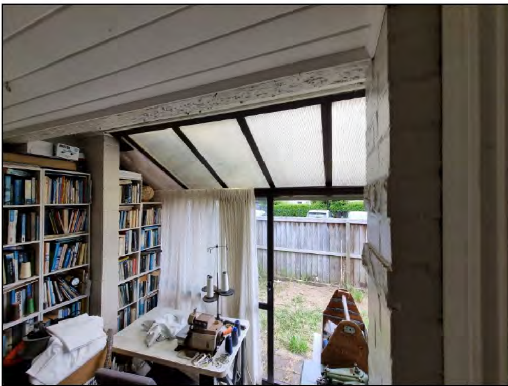
Photo 4C – Porch area used as storage.
