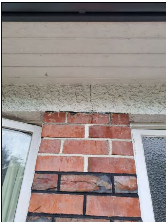
Photo 3E – Separation of the concrete beam above the cladding panel and cracking through the top brick. New mortar suggest recent cladding settlement cracks repairs along the east elevation.
