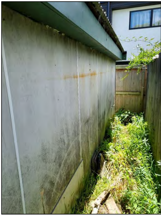
Photo 7C –Garage east elevation . Cladding is undamaged,. No stormwater guttering has been fitted.
