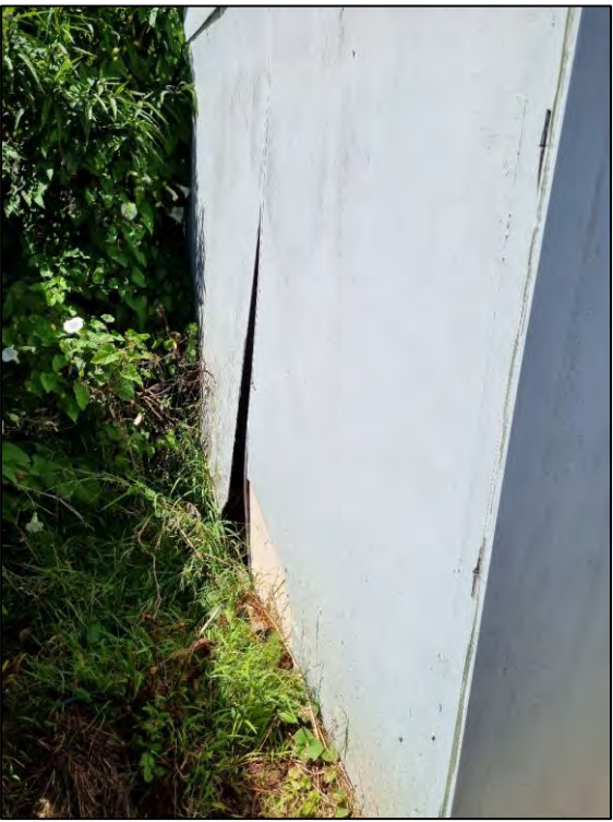
Photo 7D – North Elevation. Cladding sheet need to be refixed.
