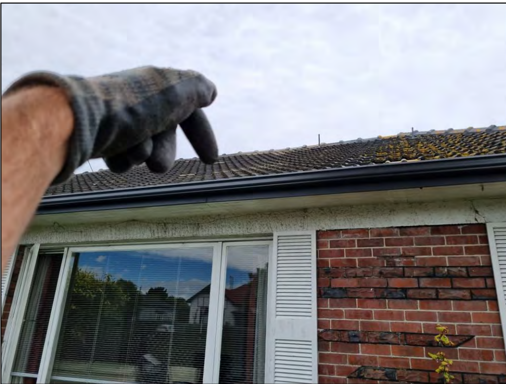
Photo 6C – Roof plane sagging towards the middle due to inadequate roof framing underpurlin support .
