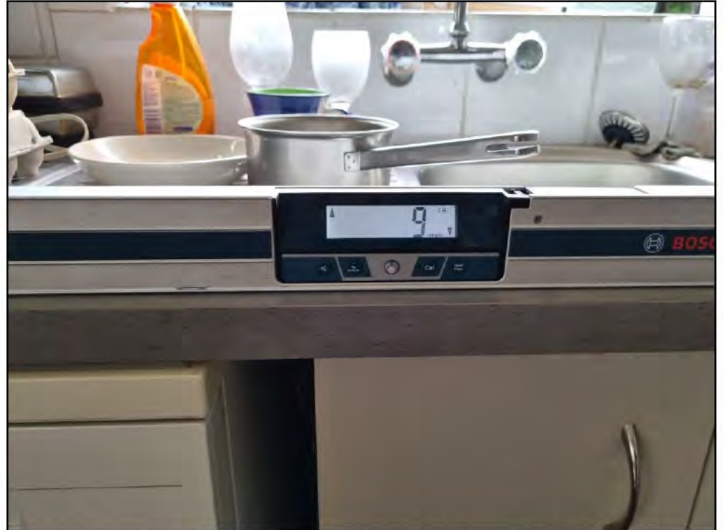
Photo 4B Kitchen bench along the eastern wall falling to the north by 9mm/m , following the floor and ceilings.
