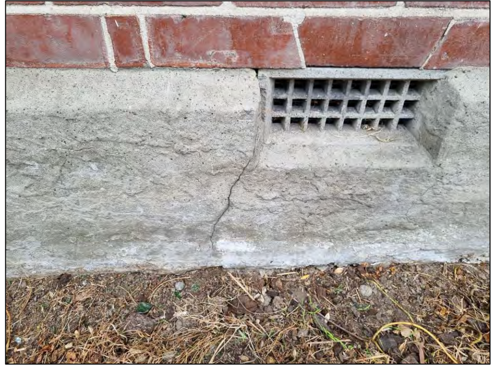
Photo 3B – Foundation crack at vent along the east elevation.
