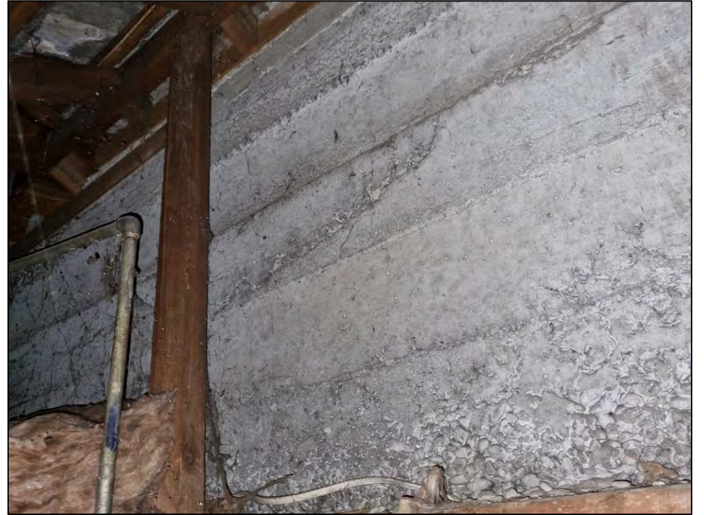
Photo 6B – Partition wall is partly constructed from poured in situ concrete above the ceiling line. Concrete pour joins ( cold joins) can be seen.
