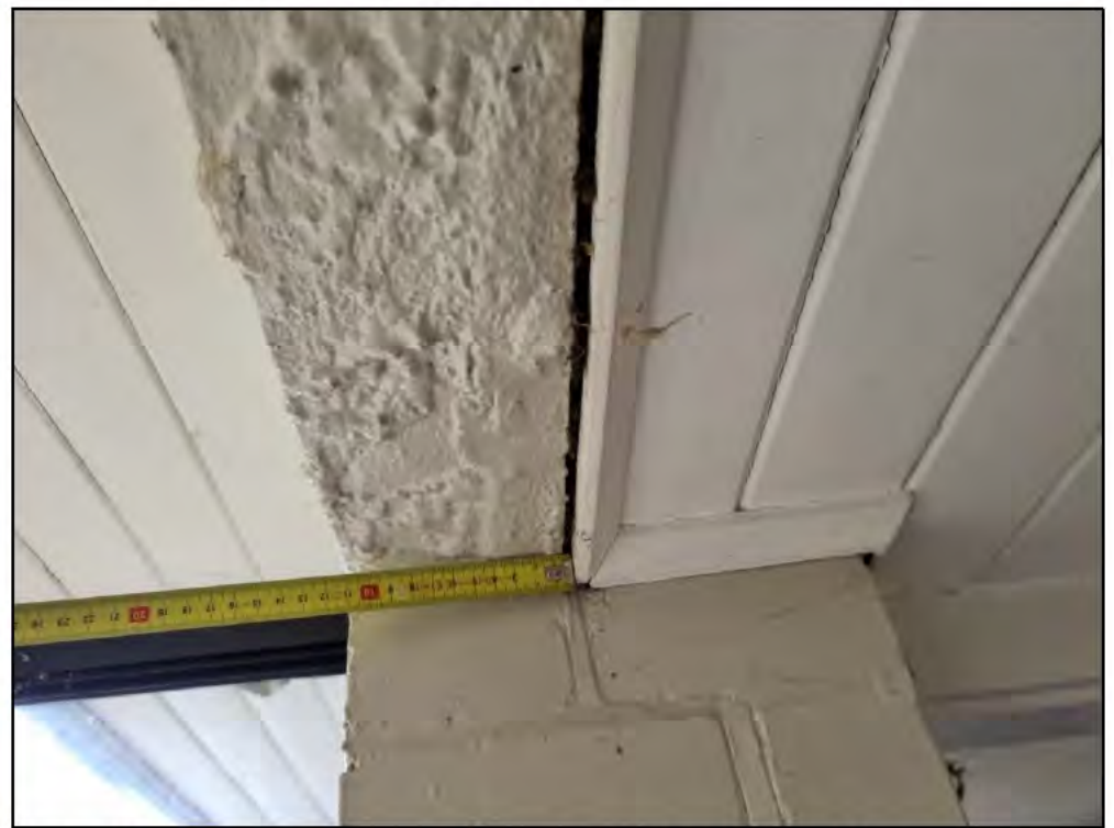
Photo 4D –Minor separation between the timber trim and the concrete lintel above the porch.
