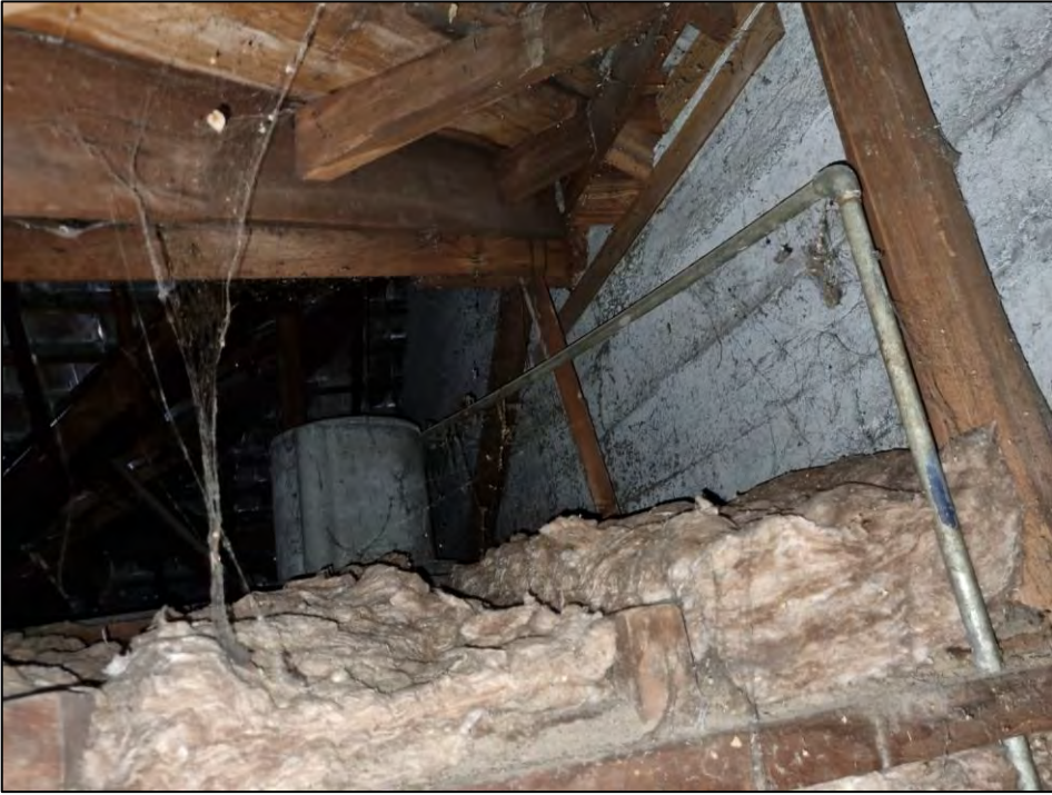
Photo 6A – Unrestrained Concrete water tank in the roof space .
