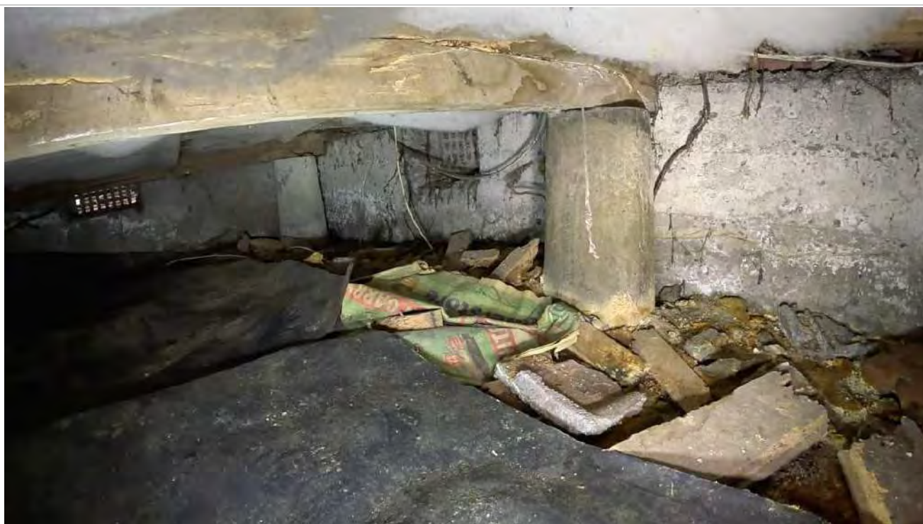
40: Precast concrete pile with no connection.
