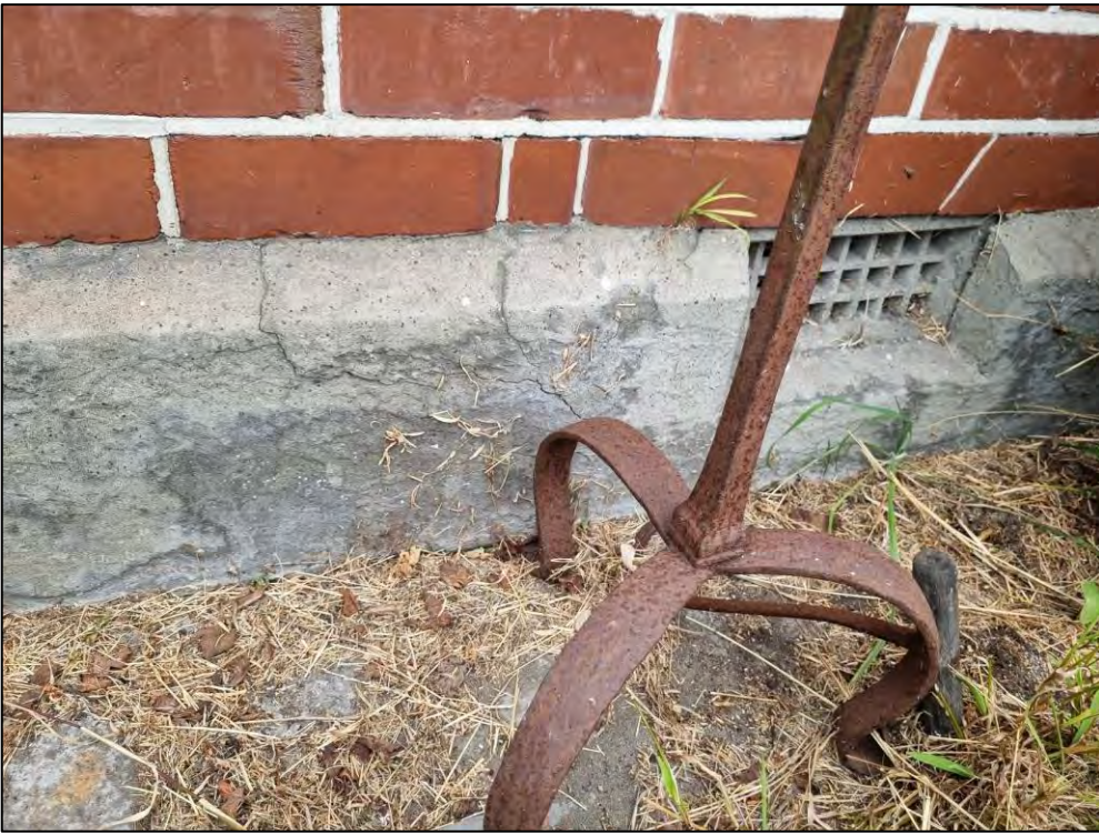
Photo 3C – Plaster and foundation cracks along the north elevation
