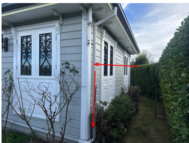
All downpipes directed into stormwater as intended
