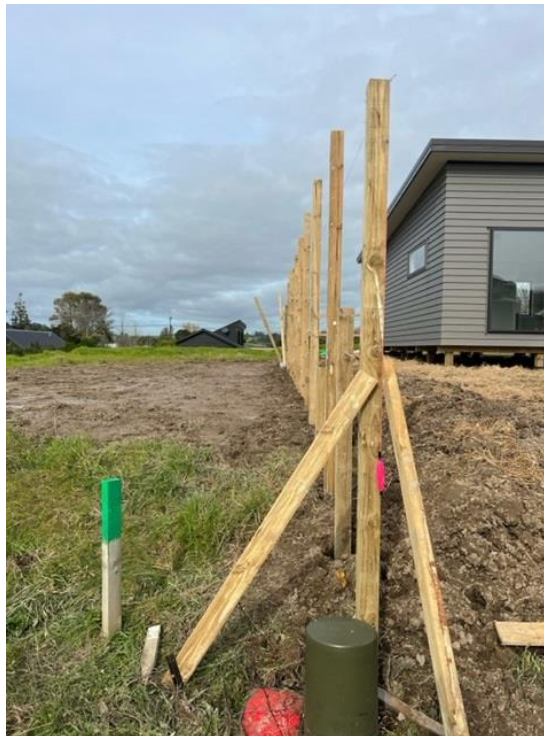
Figure 3: Western Boundary Side Setback Infringement (1.5m instead of 3m).
