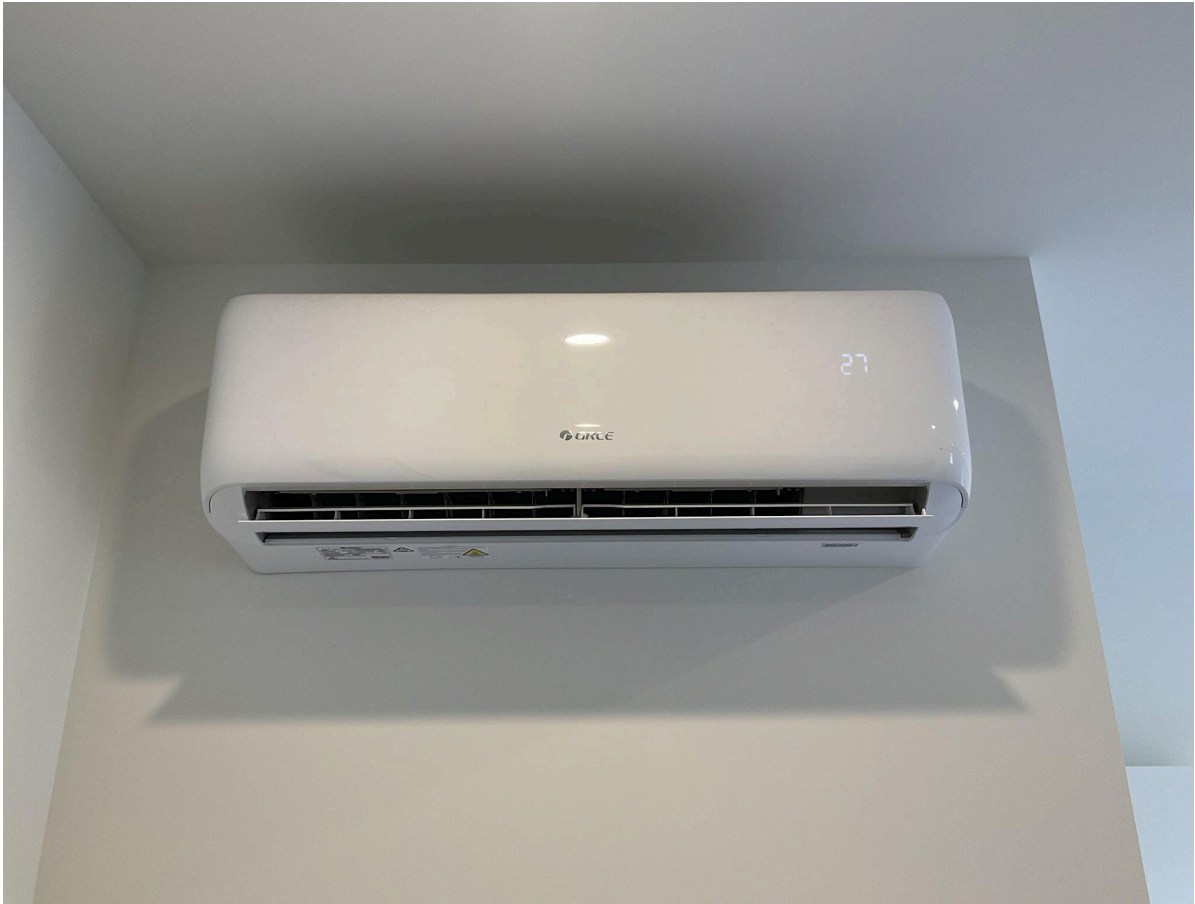
Gree high wall heat pump located in the living room 5.8KW
