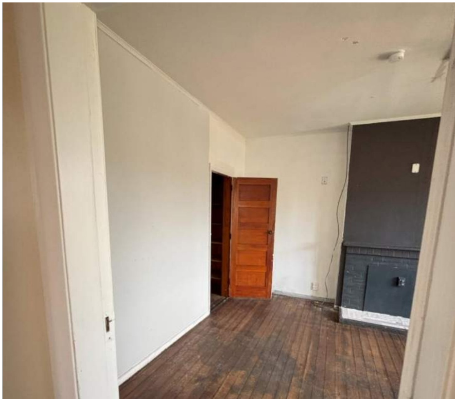
Figure 8: Internal wall within the living room of 18 Kitchener Place to be removed.
