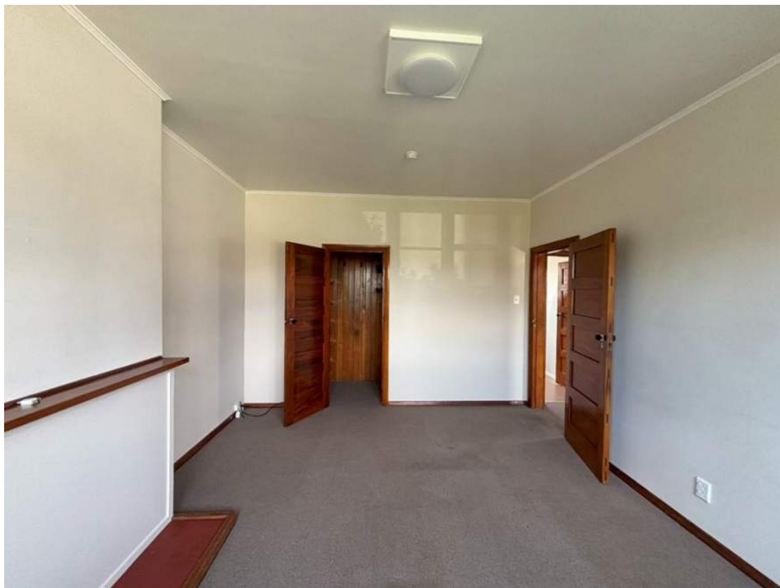
Figure 4: Internal wall within the living room of 16 Kitchener Place to be removed.
