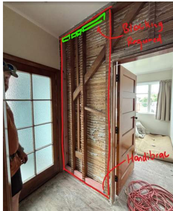
Photo 9: view of bracing wall - blocking required at top, to give space for nail fixings
