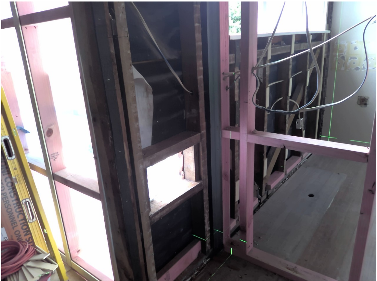
No exterior wall insulation specified , recommend insulation Taken at 12:52 PM on Friday 19/12/2025
