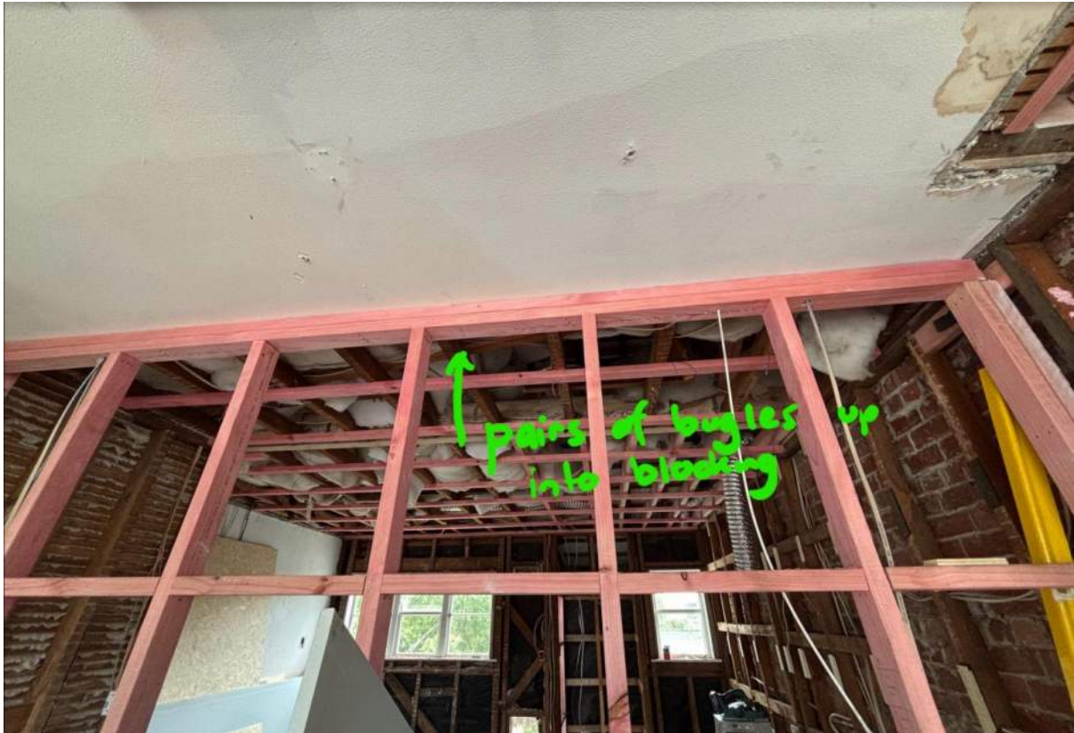
Photo 7: view of bracing wall - connection up into timber blocking via pairs of bugle screws
