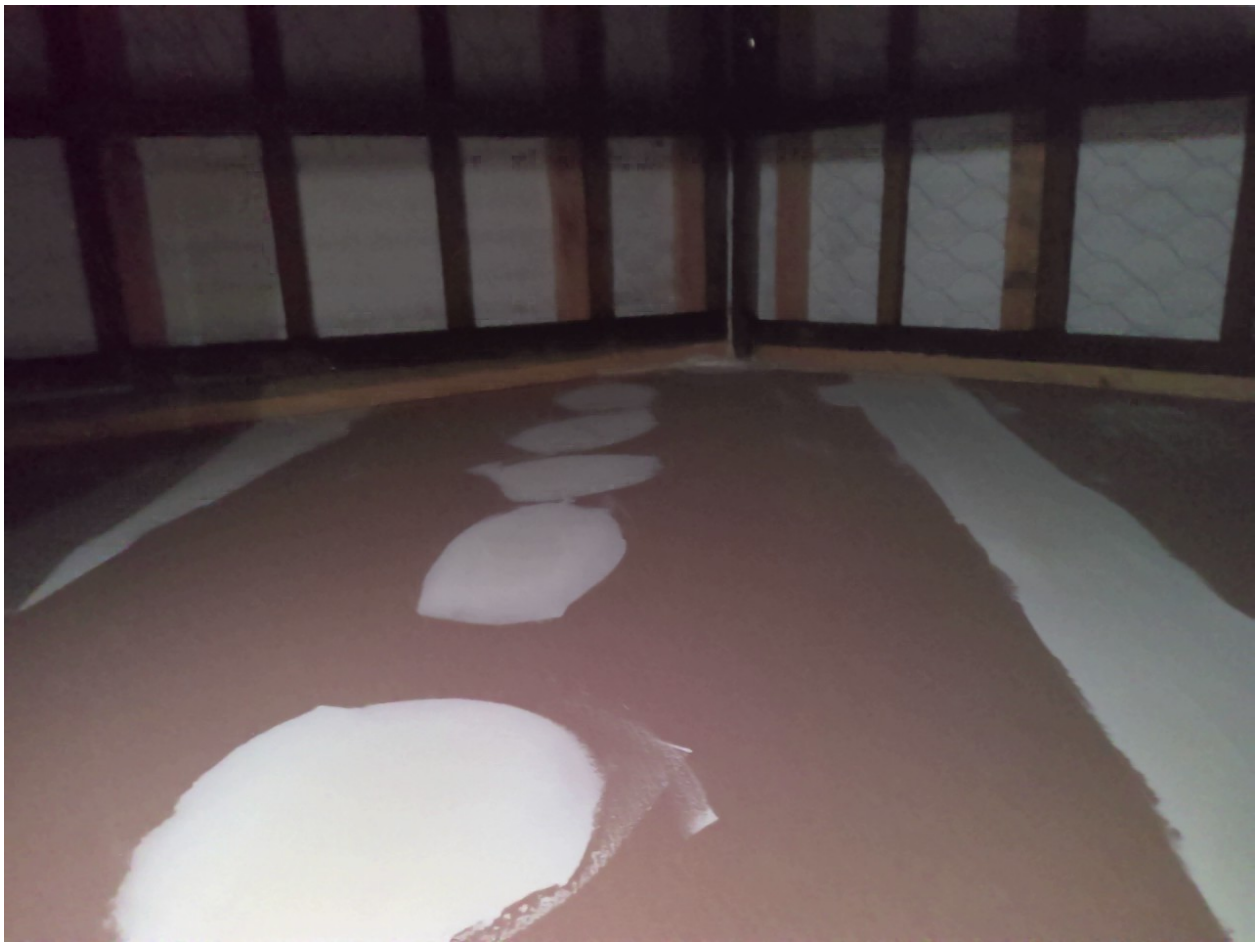
Existing FFR layers in ceiling space , on top of old brick fire wall Taken at 12:43 PM on Friday 19/12/2025
