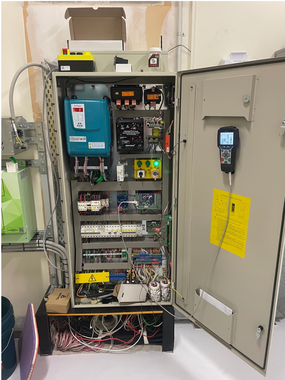
This is a new Wittur controller and what we propose to install to replace the existing 30 year old Otis MCS controllers.
