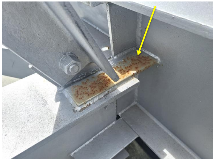
Example of corrosion to steel counterweight structure.
