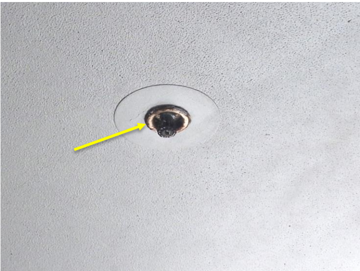
Corroded sprinkler heads to veranda soffit.
