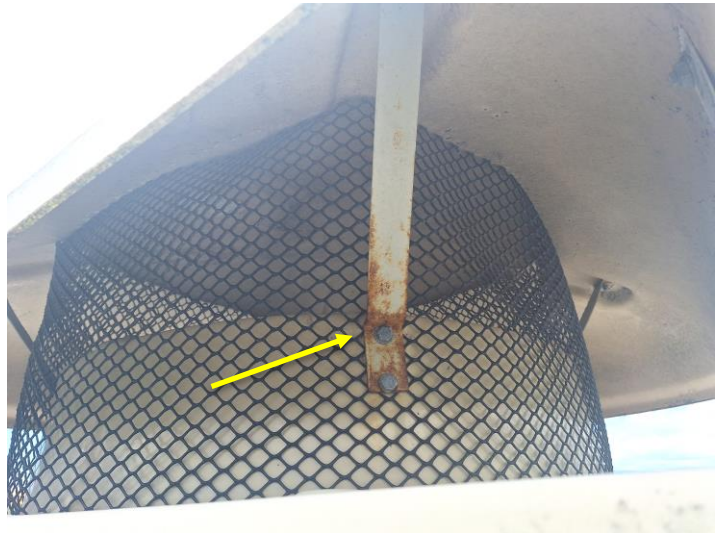
Corrosion to fan housing brackets.
