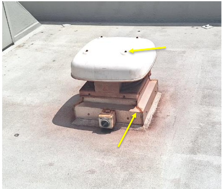
Corroded fixing screws to fan housings. Note early signs of corrosion to flashings.
