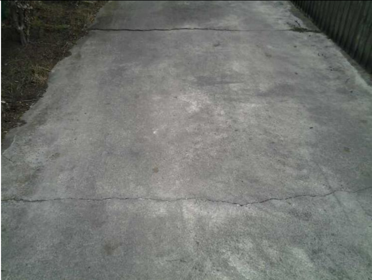
Cracks to shared drive
