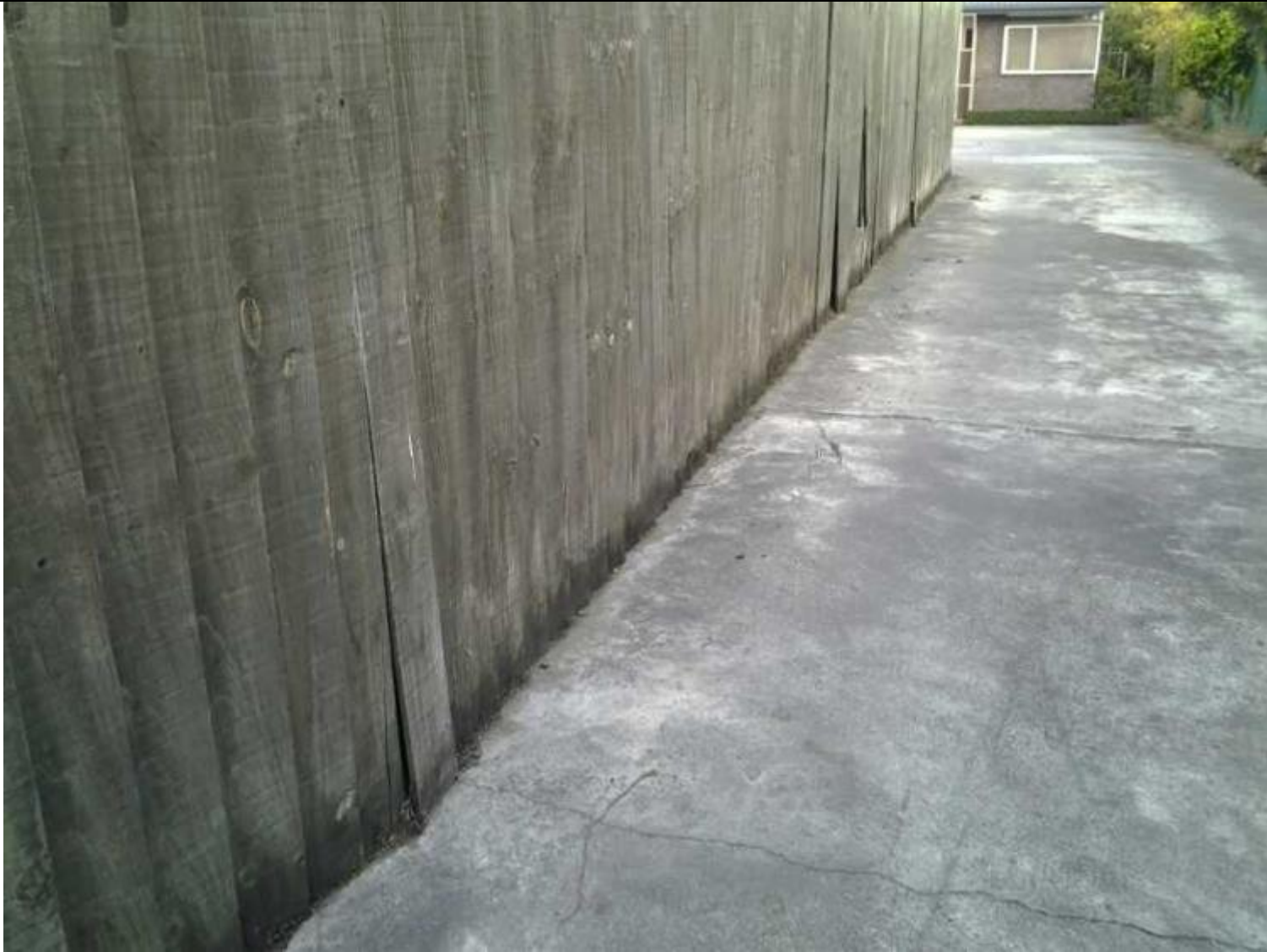
Damage to fence shared with 171a
