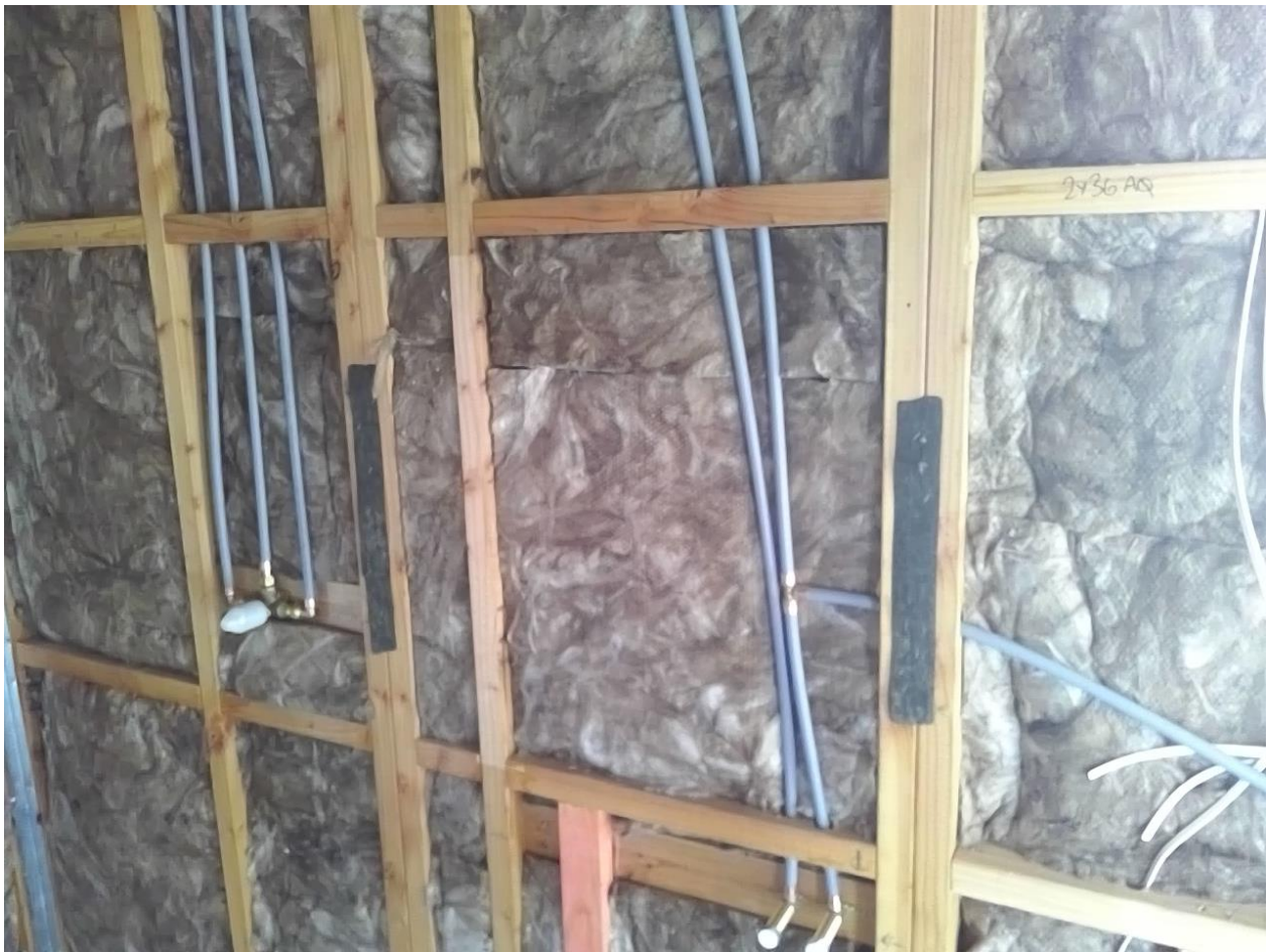
Dux Polybutylene water supply piping utilized throughout Taken at 12:27 PM on Tuesday 2/02/2021 Status: Pass
