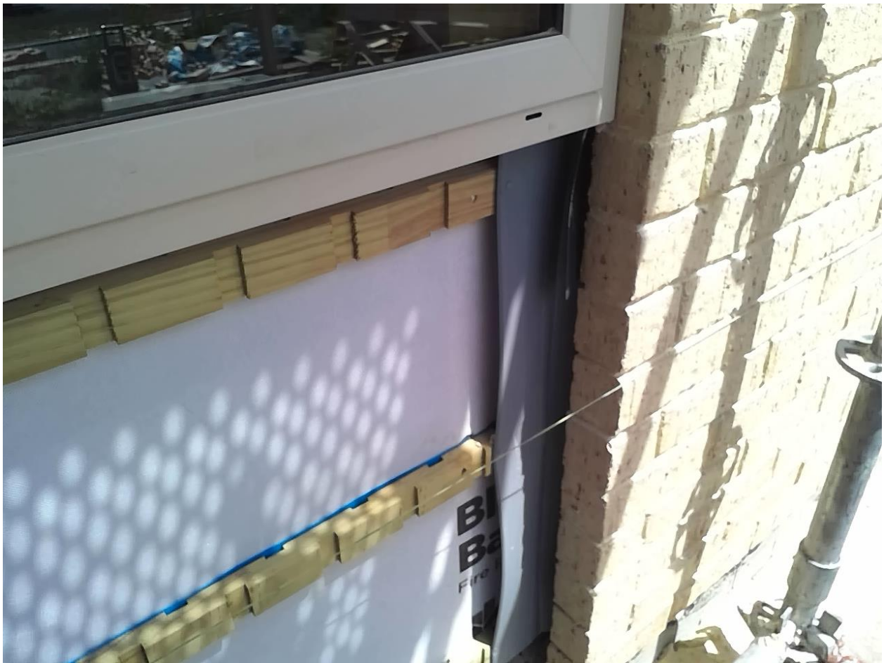
backflashing @ cladding change Taken at 12:23 PM on Monday 25/01/2021
