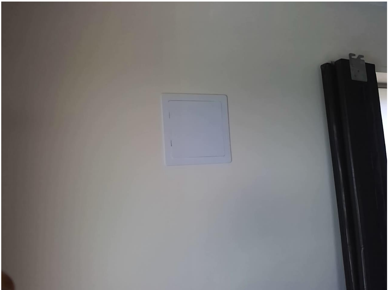
Isolation valve Taken at 1:33 PM on Tuesday 6/04/2021
