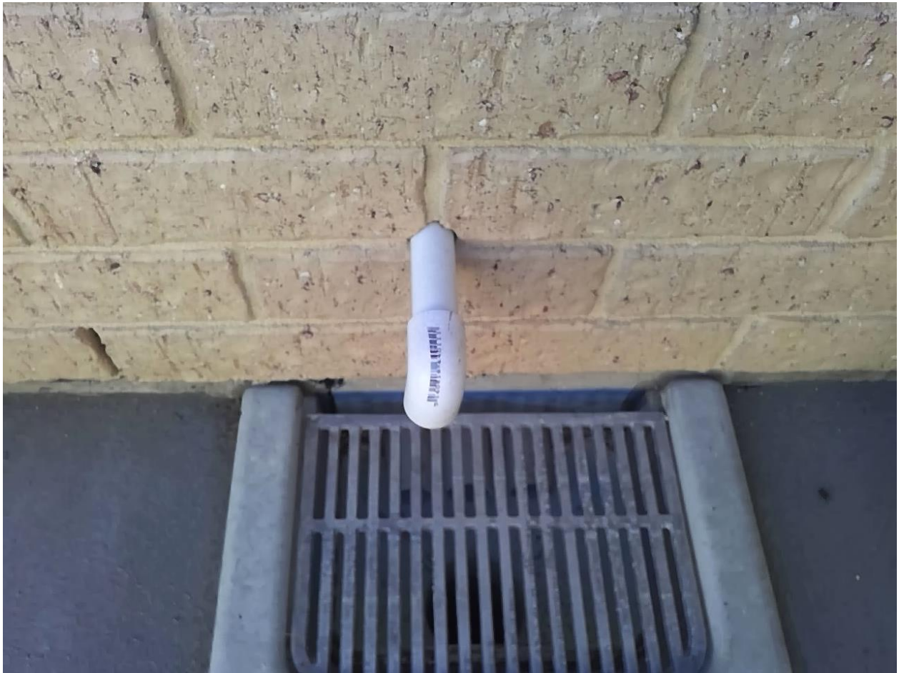
Gully trap Taken at 1:44 PM on Tuesday 6/04/2021
