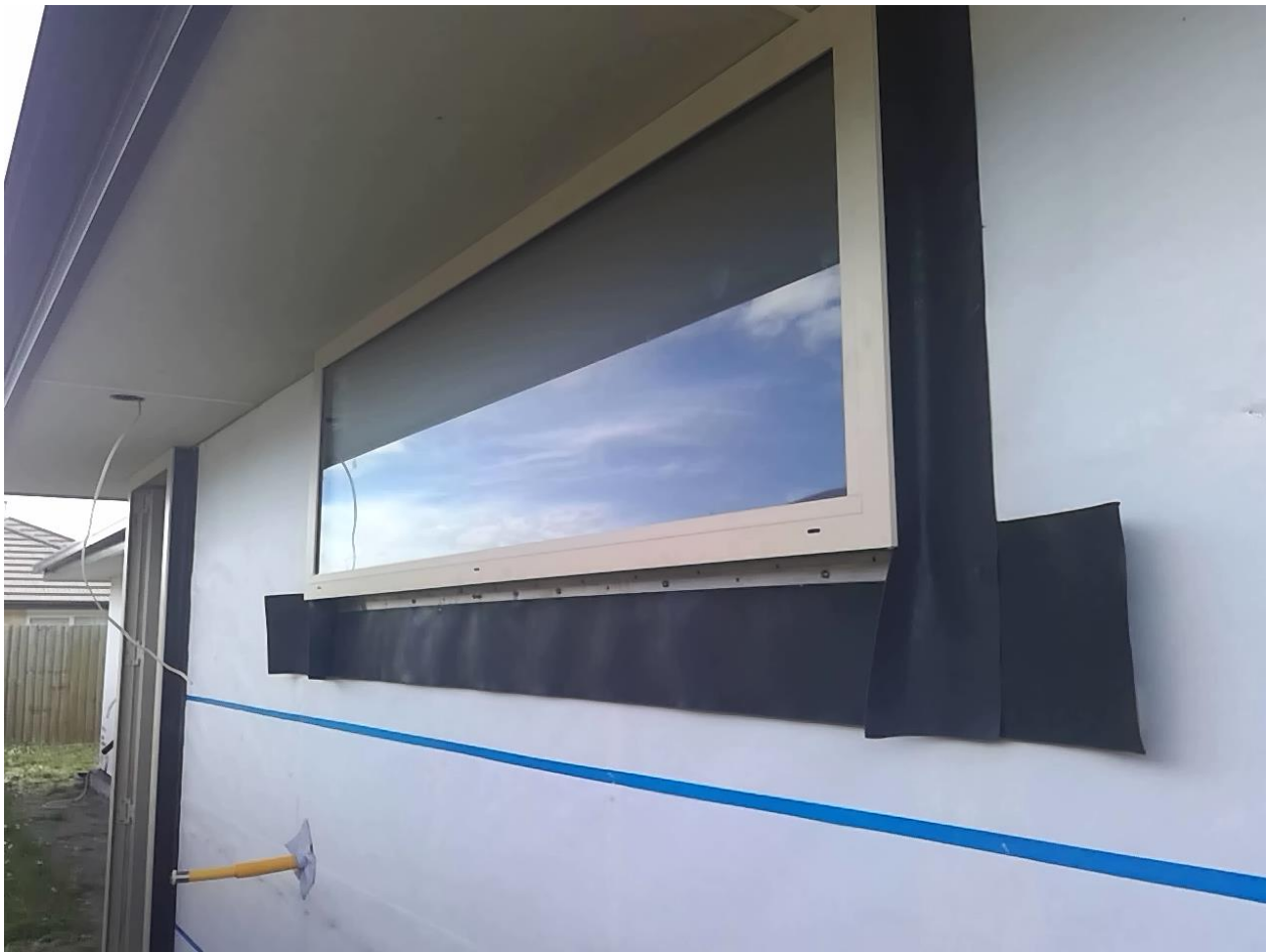
DPC flashing details to door/windows -brick areas Taken at 2:31 PM on Monday 18/01/2021 Status: Pass
