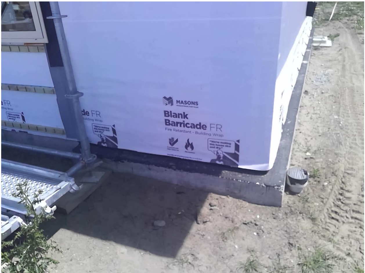
Brick rebate has been sealed Taken at 2:27 PM on Monday 18/01/2021 Status: Pass
