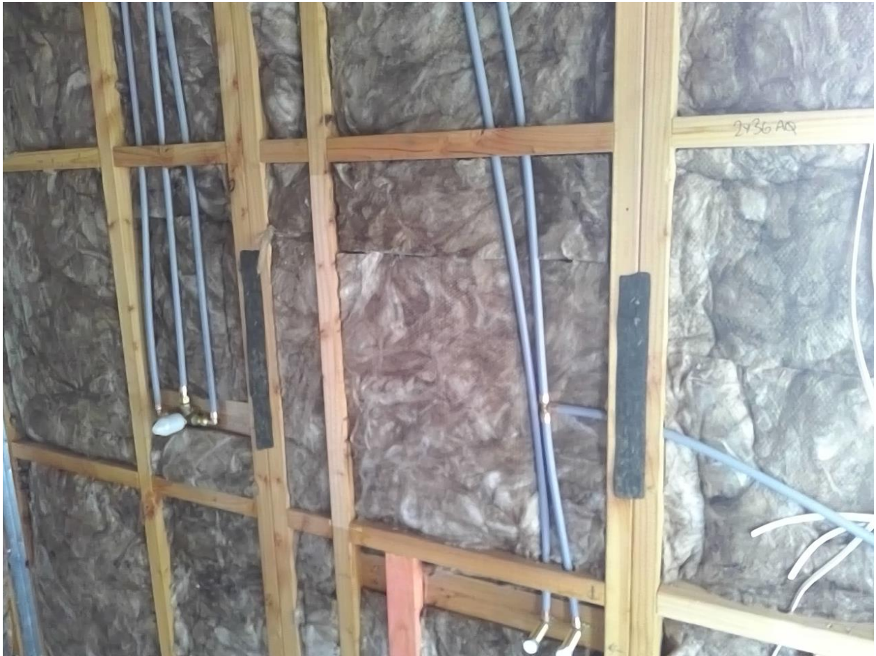
Dux Polybutylene water supply piping utilized throughout Taken at 12:27 PM on Tuesday 2/02/2021 Status: Pass
