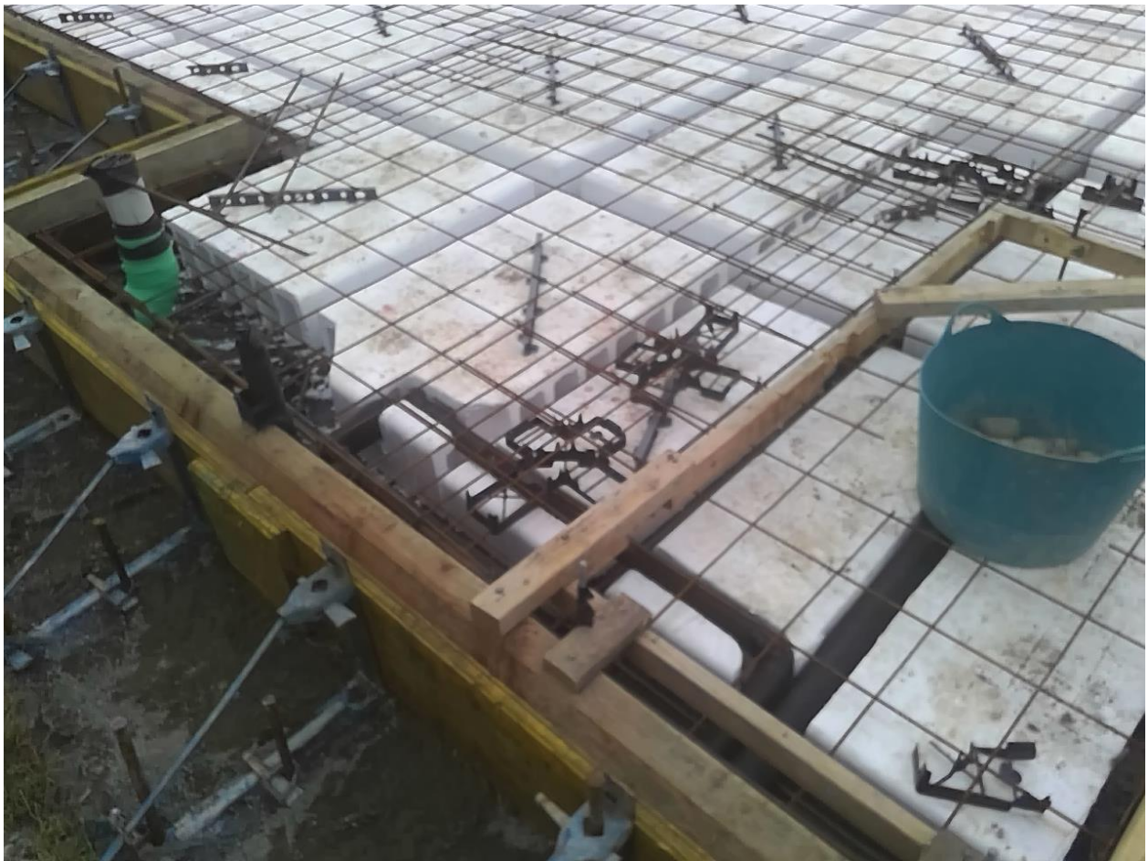
all services foam sleeved Taken at 4:13 PM on Tuesday 10/11/2020 Status: Pass
