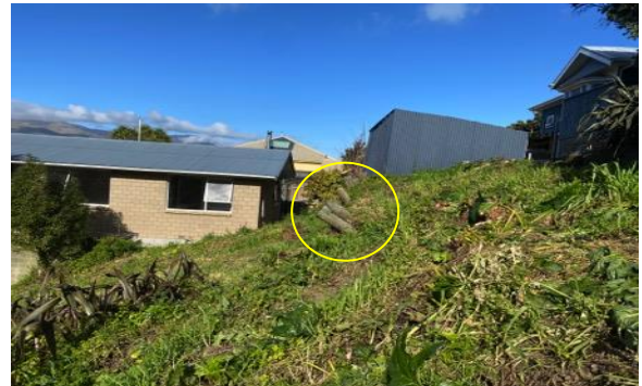
Photo 4: Looking across top (west) part of the slope towards number 4 Shackleton Tce, failed/rotated timber post retaining wall is circled.
