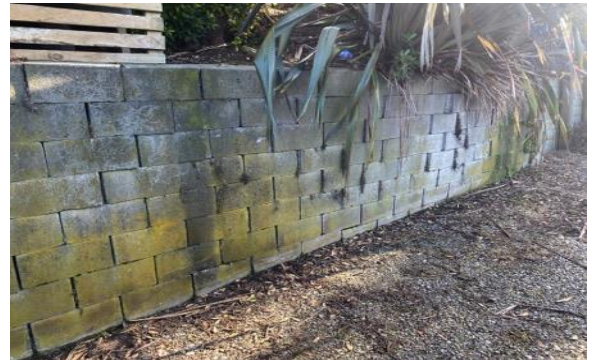
Photo 6: Loosely stacked concrete block retaining wall, west side of the site. The wall is retaining soil above the driveway
